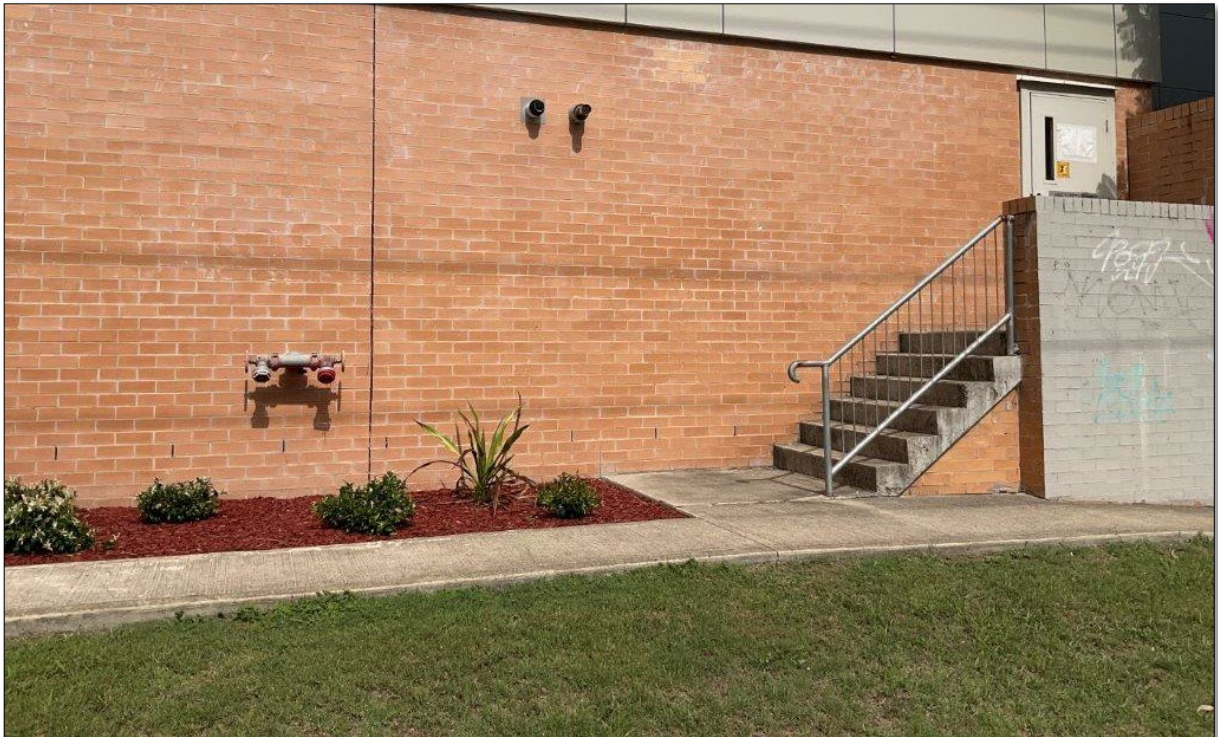
Plate 13: A double head fire hydrant is located on the northern façade of the existing building
