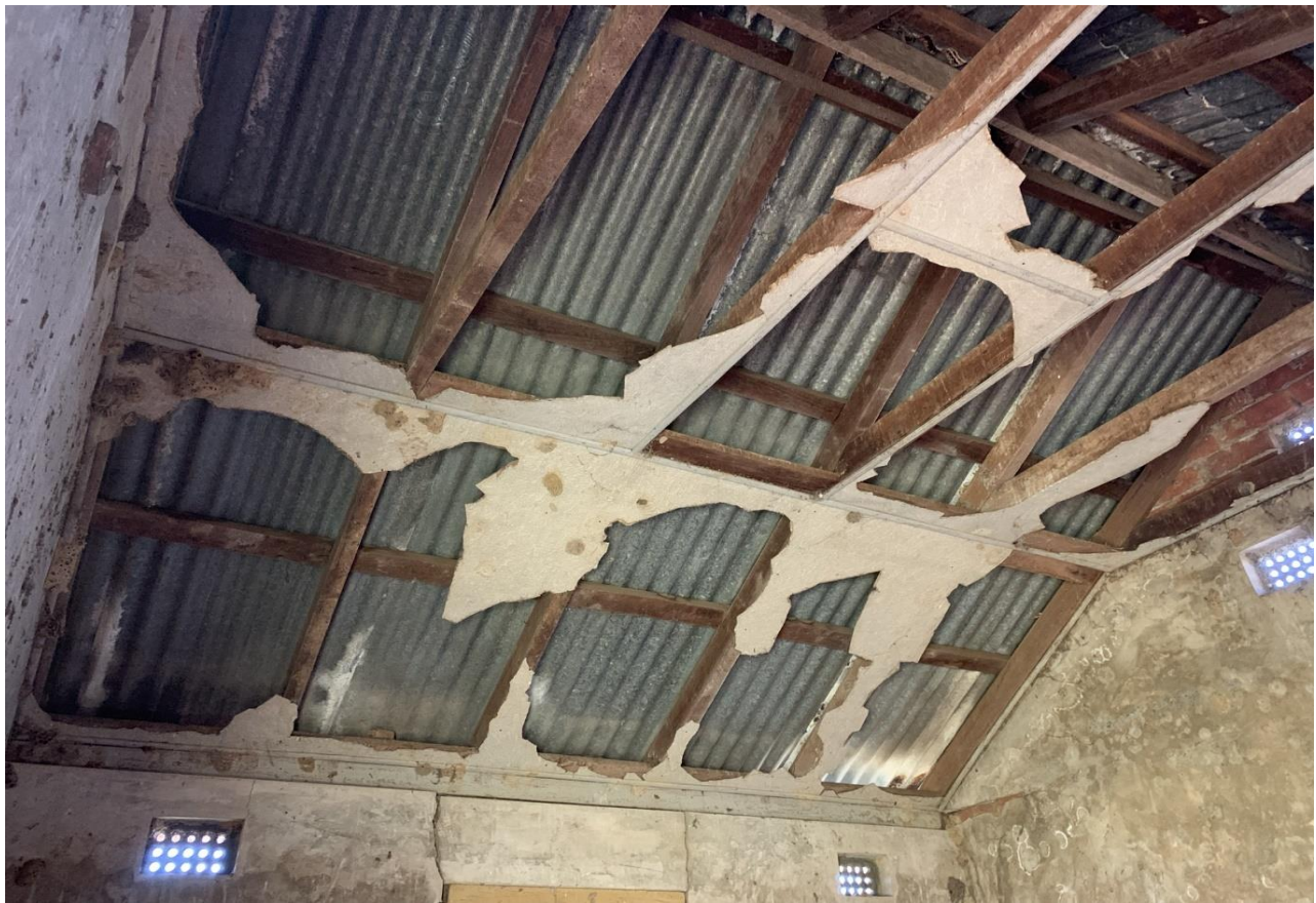
Photograph 8 - Showing possible asbestos containing roof sheeting.
