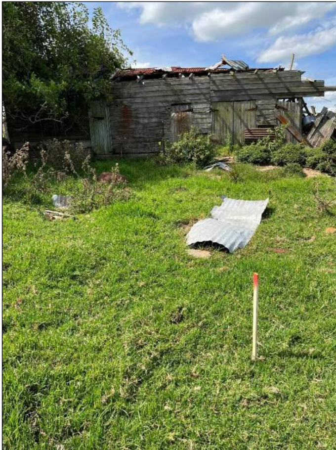
Figure 19: Former dairy structure, of timber and metal construction, in the central-southern portion of the site, looking north
