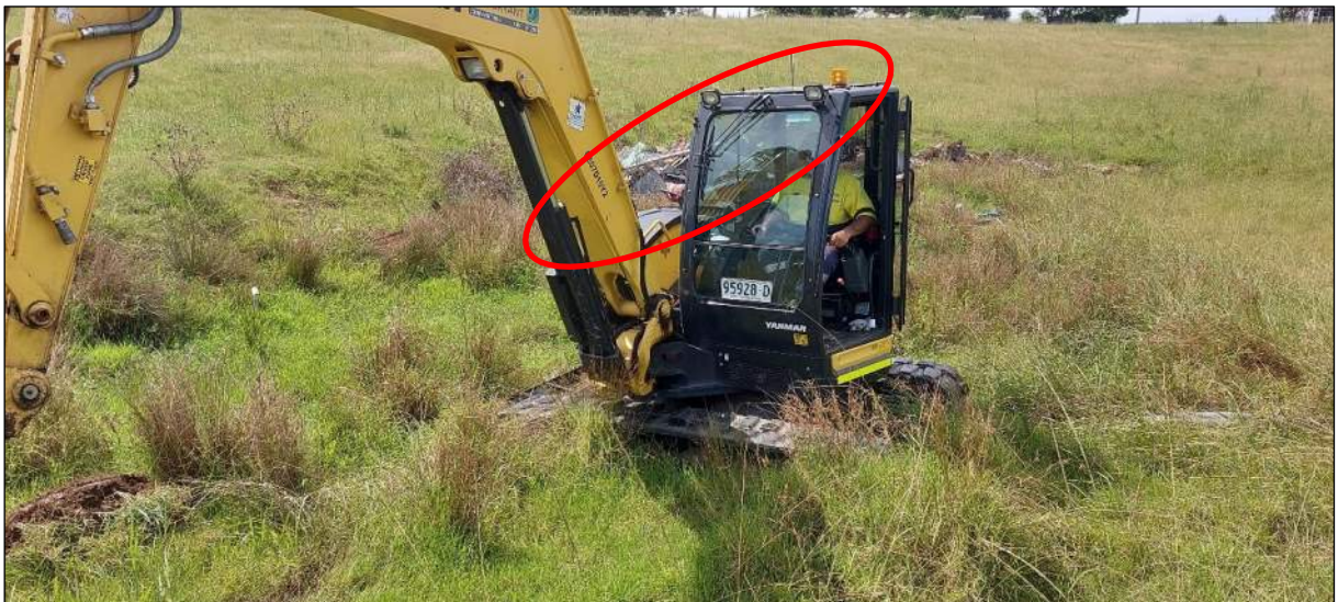
Figure 25: Infilled dam (red circle) in the central-southern portion of the site, looking north
