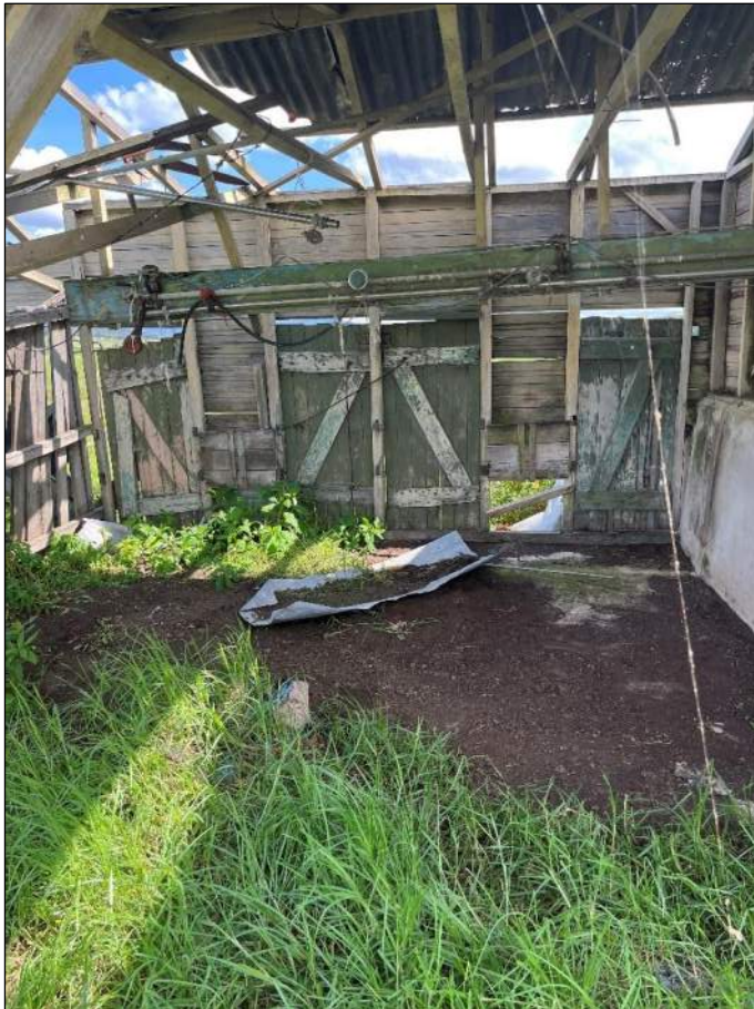
Figure 20: Former dairy structure, of timber and metal construction, in the central-southern portion of the site, looking south
