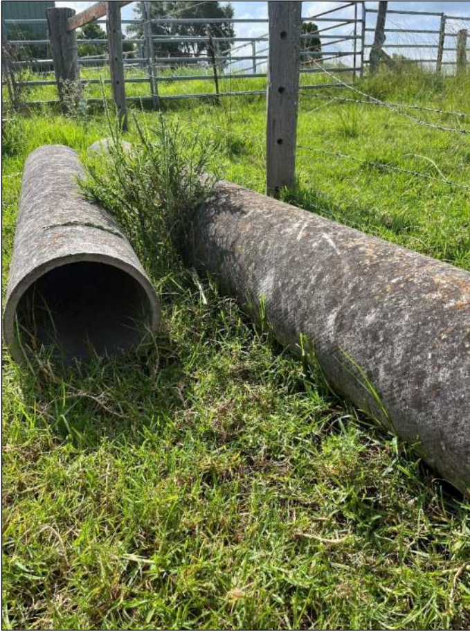
Figure 24: Cement pipes (possible asbestos containing materials) in the central-southern portion of the site (i.e. former dairy area)
