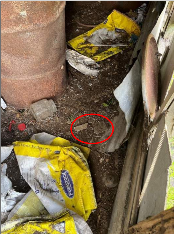
Figure 21: Cement sheeting/cladding on the walls of a portion of the former dairy, with some broken sheeting on the exposed soil (in red circle) in the central-southern portion of the site.
