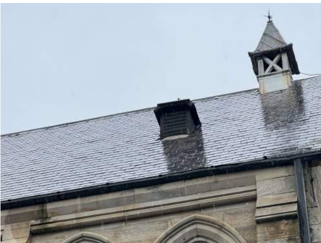
Figure 25 Detailed view of slate roof with timber dormers and bellcote. source: Heritas, 2022.
