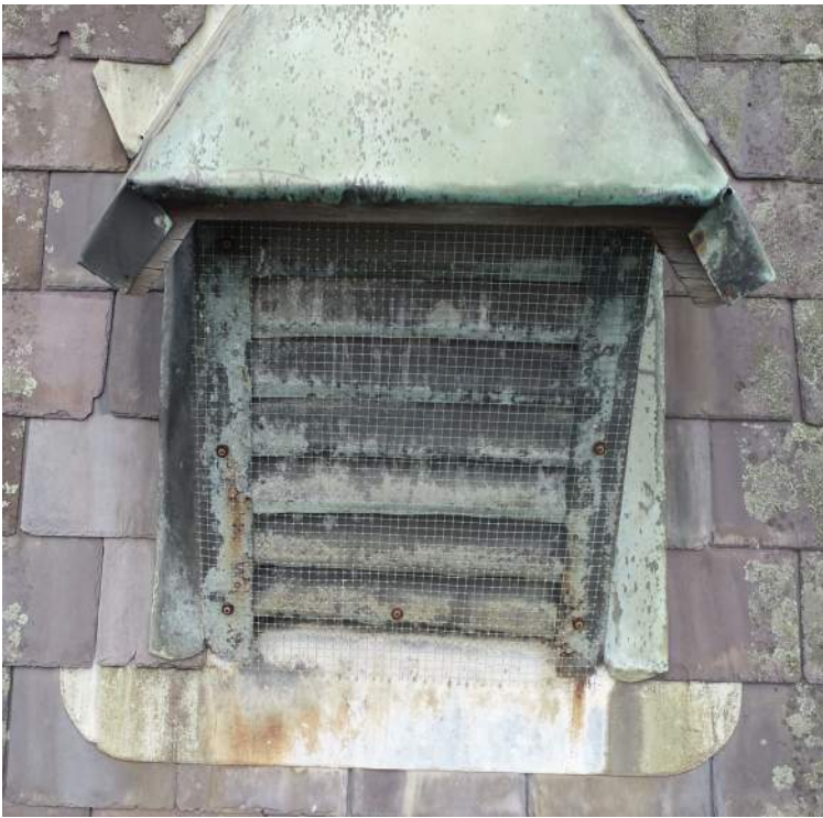
Figure 36 View of timber framed dormer with copper roof cladding and flashing. Copper louvres in poor condition. source: iScope Consultants, March 2021.
