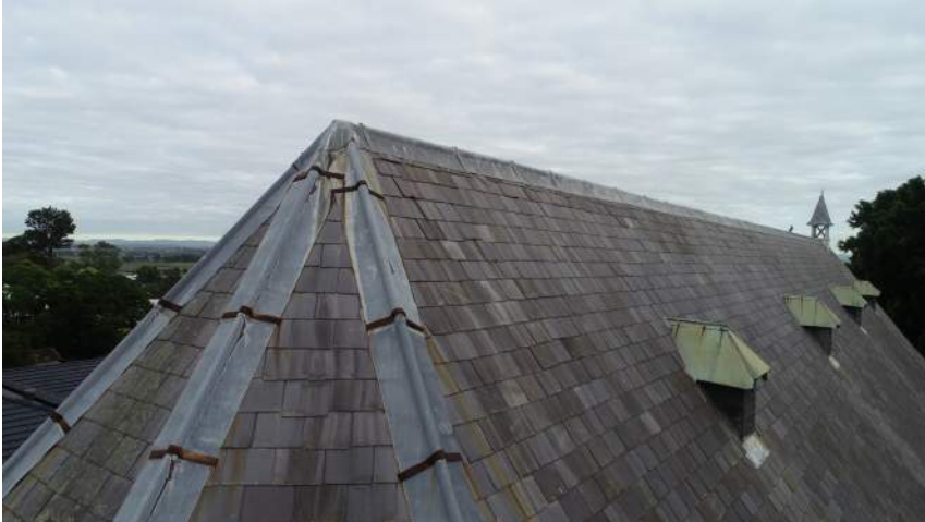
Figure 29 Aerial view of metal ridge capping impacted by hail damage. Note also the condition of the dormer cladding. source: iScope Consultants, March 2021.
