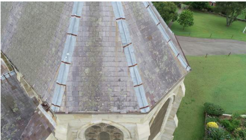
Figure 30 Aerial view of metal ridge capping and guttering impacted by hail damage. source: iScope Consultants, March 2021.
