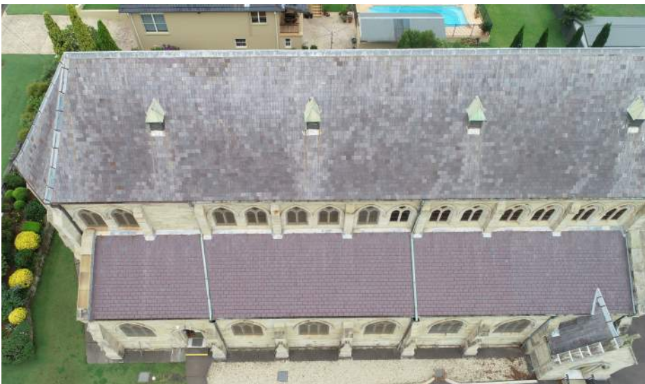
Figure 28 Aerial view of slate roof to church. Slate replaced to north aisle. Note difference in condition of slate. source: iScope Consultants, March 2021.
