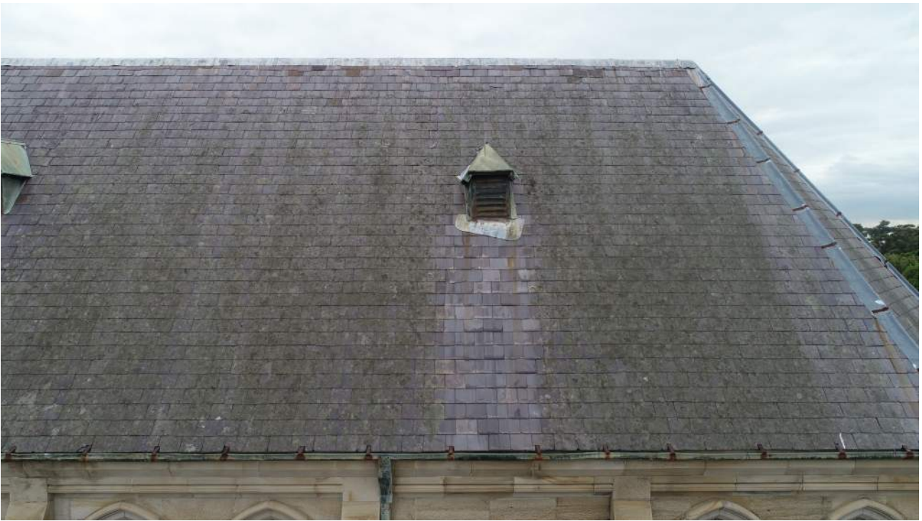
Figure 32 View of damaged dormer with metal cladding, metal louvres and flashing in poor condition. source: iScope Consultants, March 2021.
