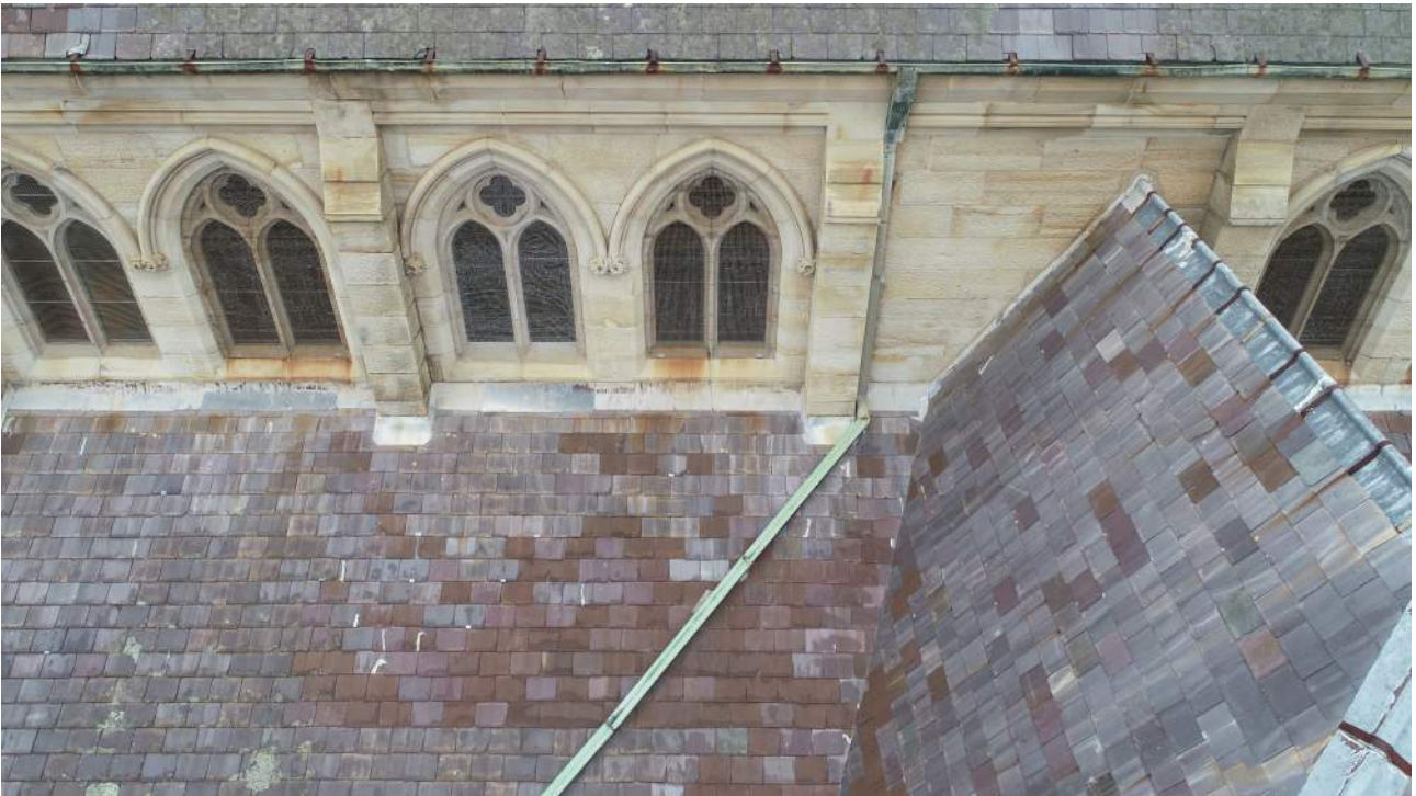
Figure 33 View of metal gutter in poor condition with new slate tile repairs evident to lower roof plane. source: iScope Consultants, March 2021.
