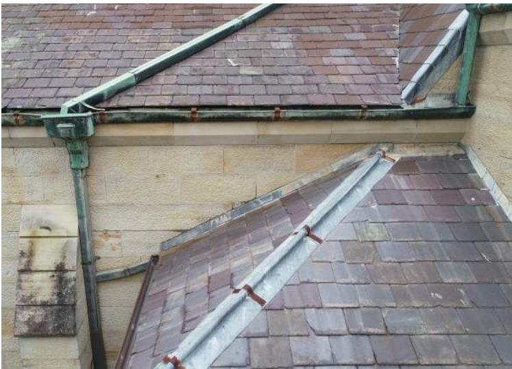
Figure 37 Detailed view of copper rainwater heads and metal guttering in poor condition. source: iScope Consultants, March 2021.
