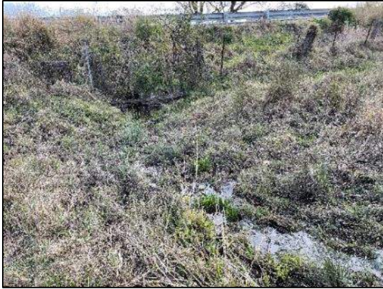
Plate 13: Left Segment ID 1.7 Culvert showing no defined bed or bank along eastern side of Cessnock Rd facing west.
