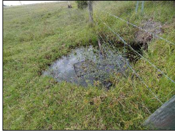
Plate 14: Right Segment ID 1.7 (right) Culvert on western downstream side of Cessnock Rd.
