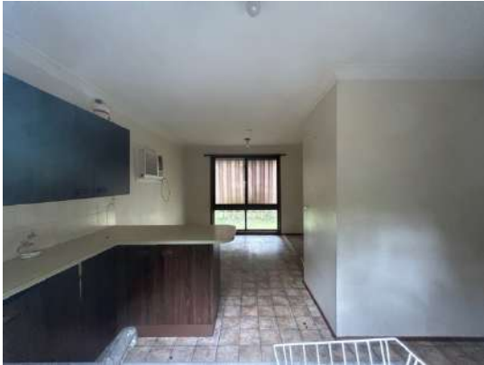
Open plan kitchen through to front dining and living space. Overall Condition: Poor
