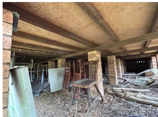
Subfloor space showing particle board flooring over timber bearers and joists on brick piers.
