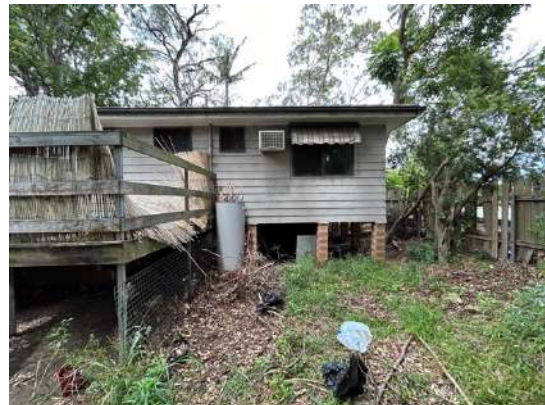
The rear of the dwelling showing brick piers and fibre-cement weatherboard cladding.
