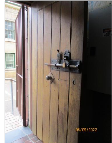
Figure 69 Typical cell door bolt and lock. This lock is one of the more recent Abloy Lock types.
