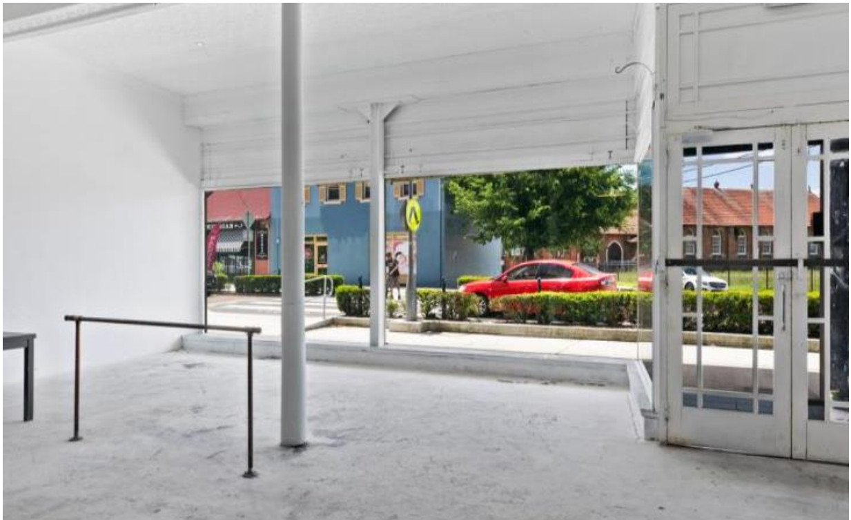
Figure 3 – Internal layout of the ground floor of the existing food and drink premises
