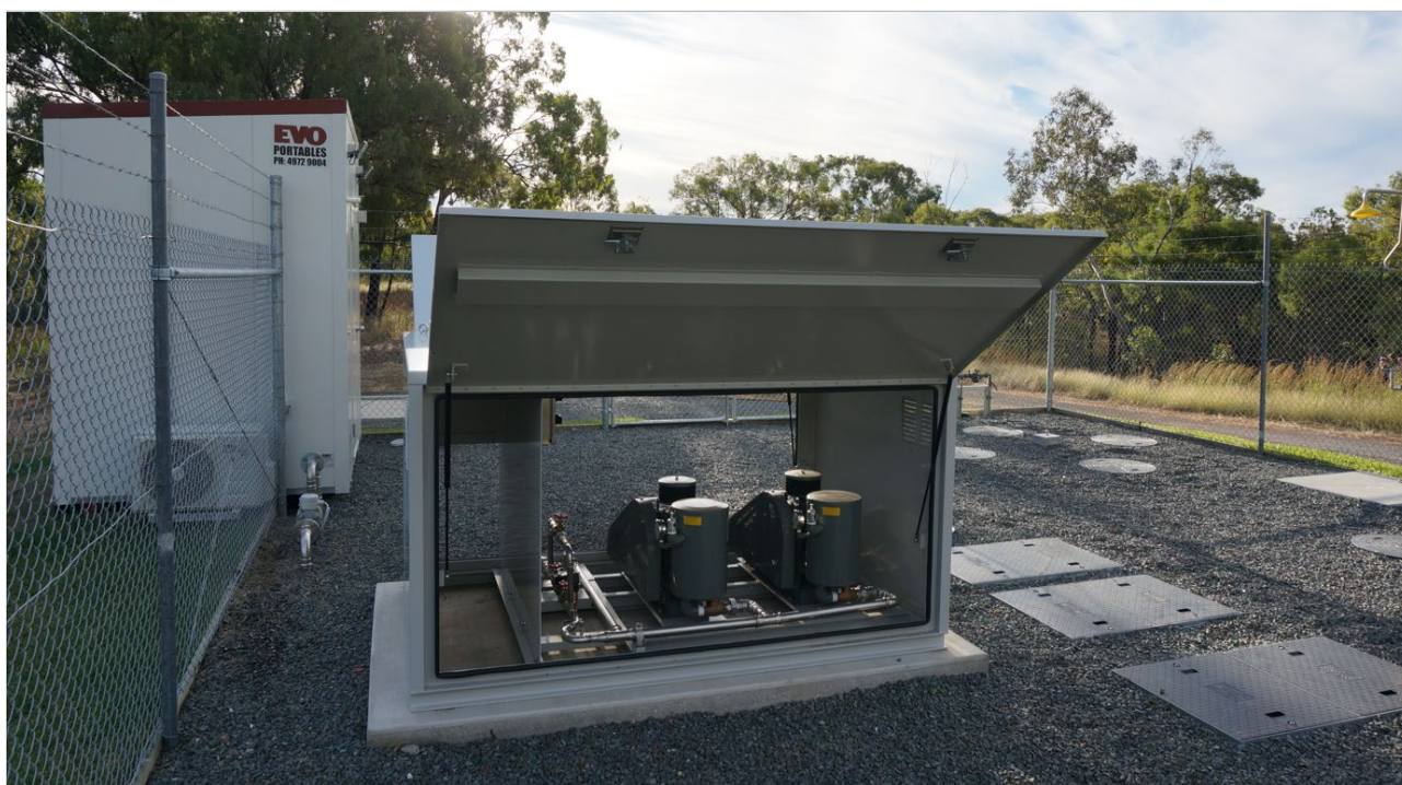
Figure 9.4 – 40kL Kubota WWTP for Water Utility - Plant room, electrical box, and monitoring unit (foreground) site office (background)
