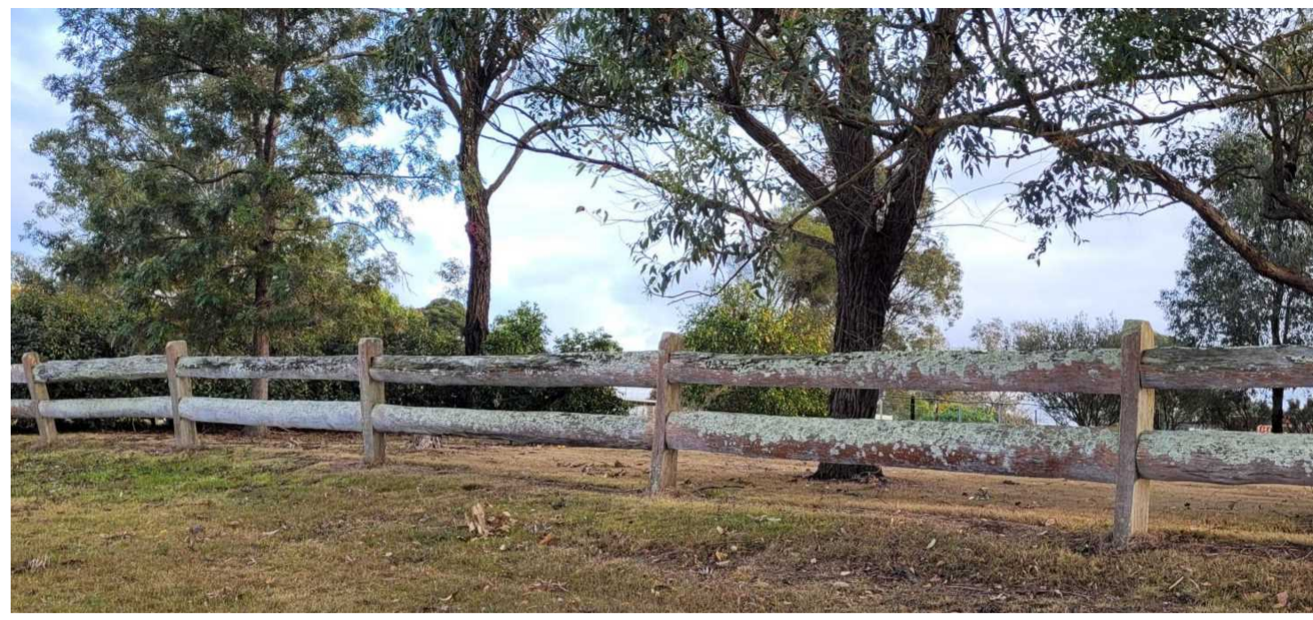
Post and rail fence on front boundary to continue post and rail fence on opposite side, and adjacent fence to east.
