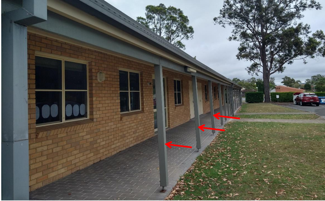
Photograph 9: Block B, exterior, awning posts and beams, green paint, non-lead paint (≤0.1% lead w/w)
