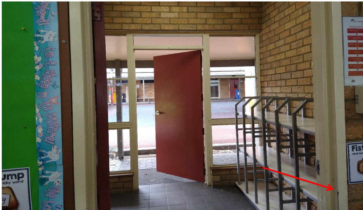
Photograph 2: Block B, B1 - interior, internal door frame, cream paint, non-lead paint ( \leq 0.1\% lead w/w)
