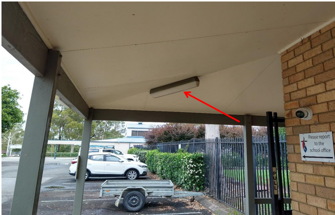
Photograph 12: Block B, exterior, eaves/ awnings, fluorescent light fittings, PCB (suspected)
