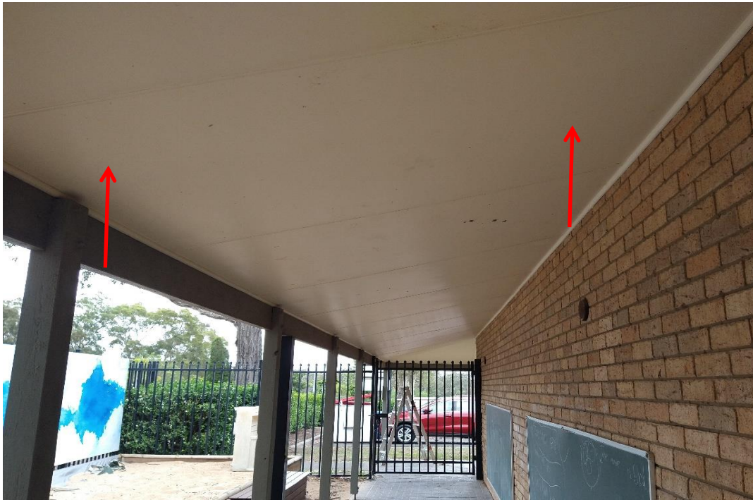
Photograph 10: Block B, exterior, awning lining, fibro sheeting, no asbestos detected by analysis
