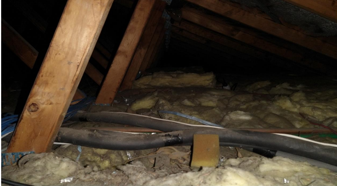
Photograph 7: Block B, B2 - interior, ceiling / roof space (Room B2), settled dust / debris, elevated lead (11mg/m2)
