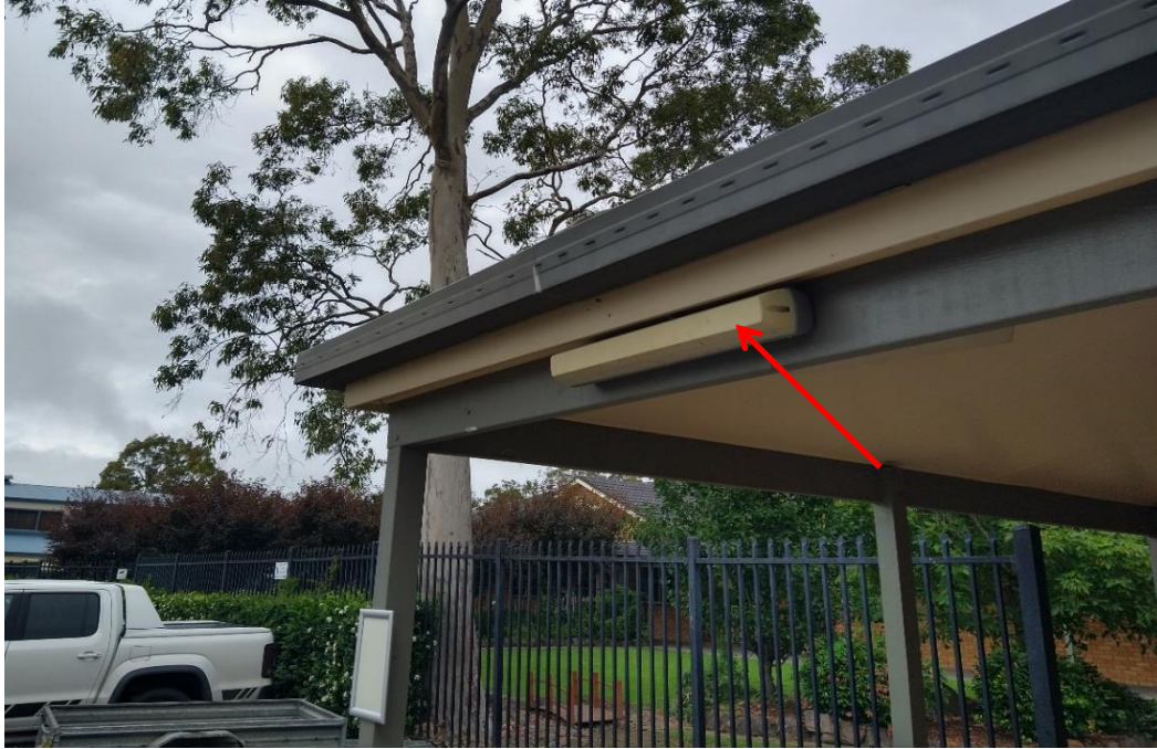
Photograph 15: Block B, exterior, eaves/ awnings, fluorescent light fittings, PCB (suspected)
