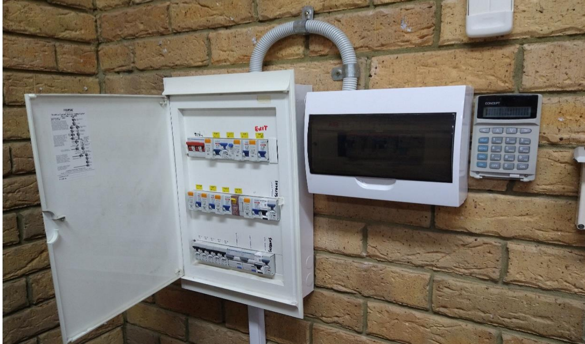
Photograph 13: Block B, B3 - interior, electrical distribution board, plastic backing board, nil asbestos
