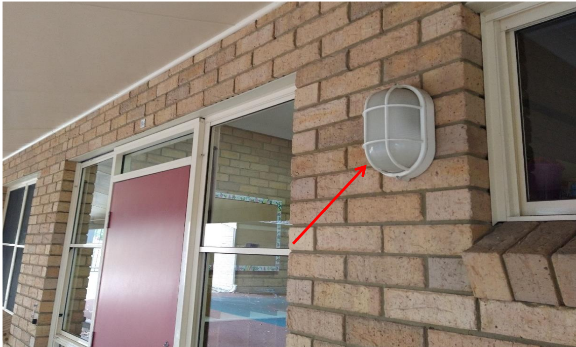
Photograph 14: Block B, exterior, eaves/ awnings, fluorescent light fittings, PCB (suspected)
