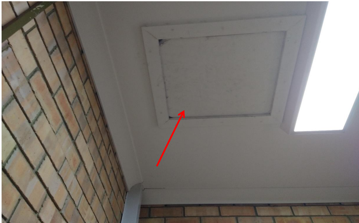
Photograph 5: Block B, B2 - interior, ceiling / roof space (Room B2), settled dust / debris, elevated lead (11mg/m2)
