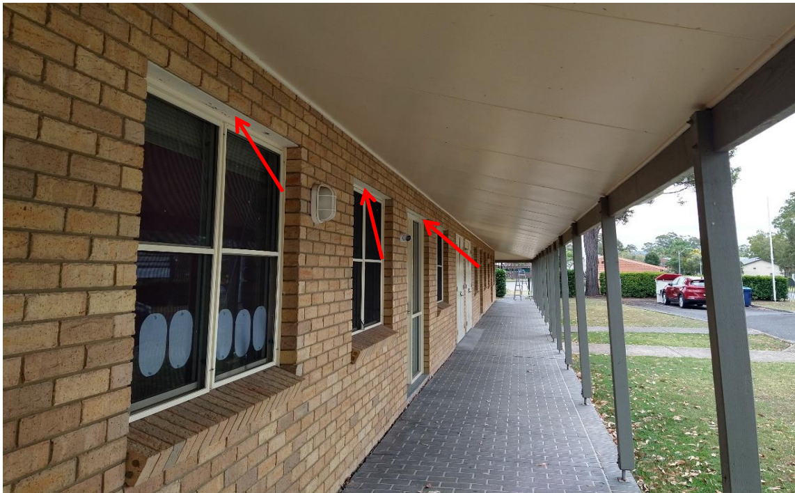
Photograph 8: Block B, exterior, external door and window frames and lintels, cream paint, lead paint (>0.1% lead w/w)
