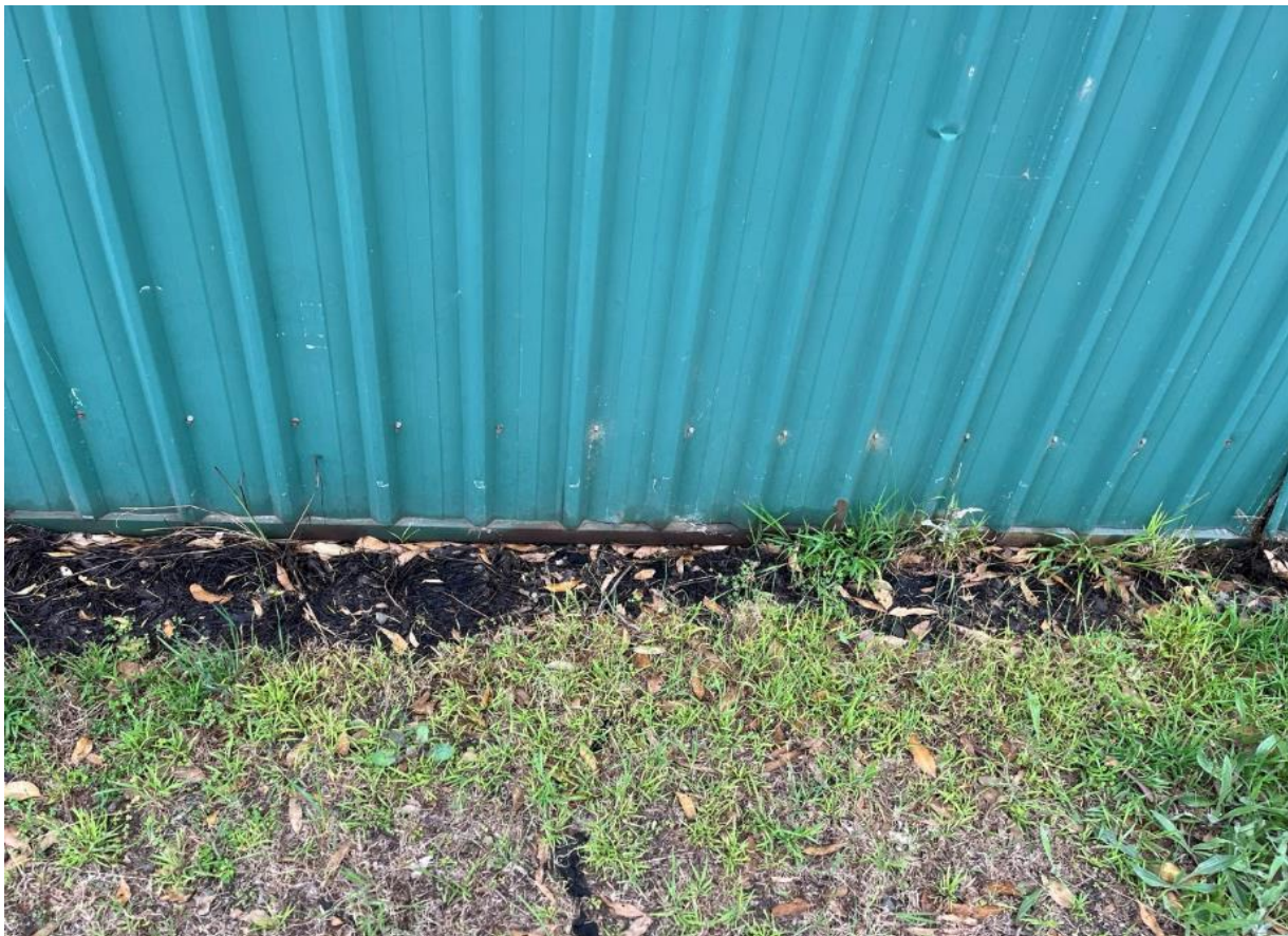
Photograph 30 - Staining observed on southern wall of Shed 4 - 10 River Road.
