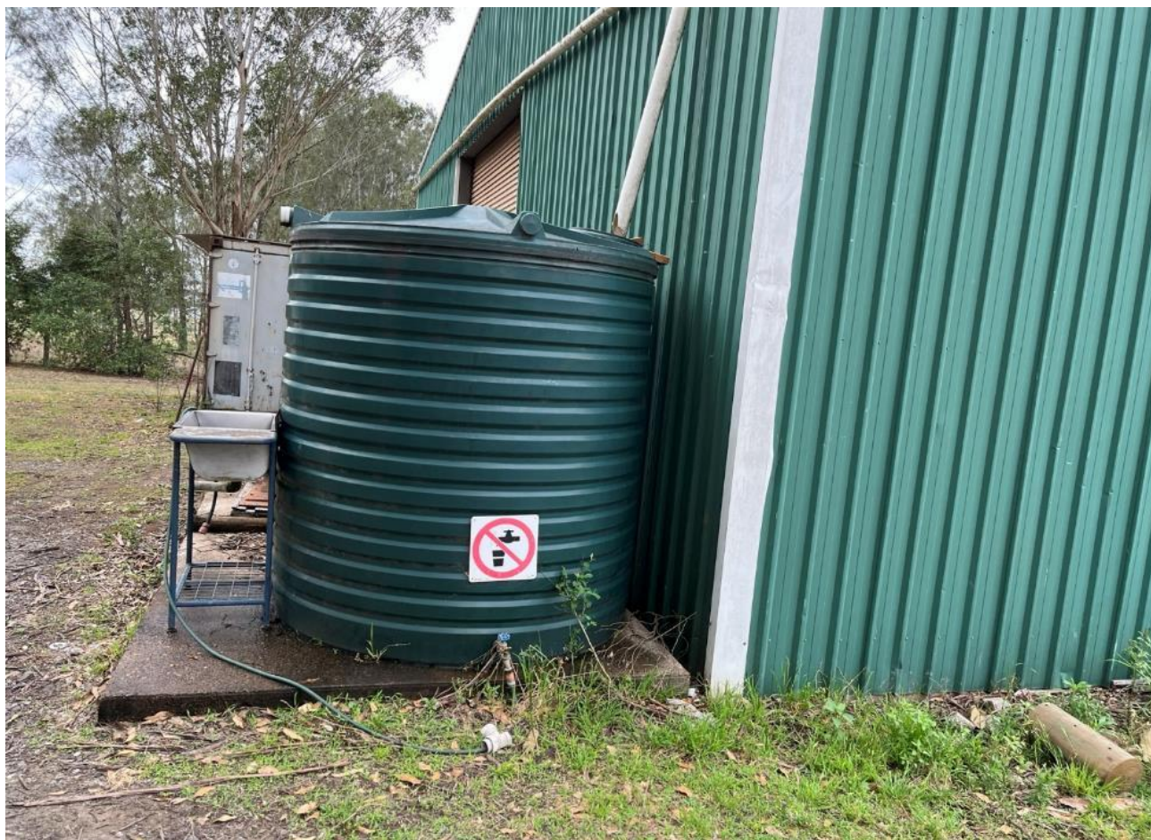
Photograph 32 - Rainwater tank on northern wall of Shed 4 - 10 River Road.
