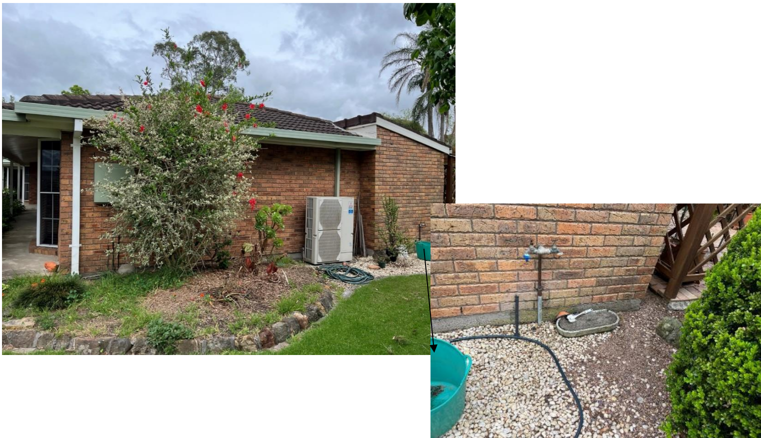
Photograph 2 - Dwelling 1 air con unit and grease trap - 10 River Road.
