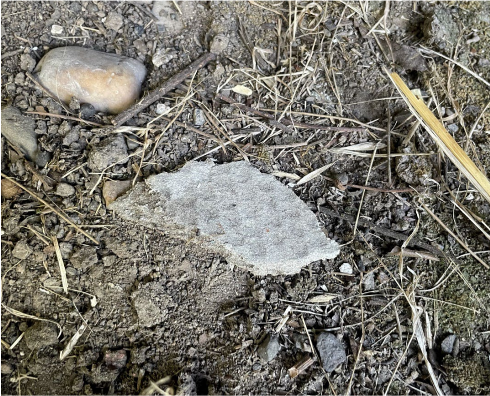
Photo 13: Potential Asbestos Containing Material (PACM) sample taken from underneath the dwelling.
