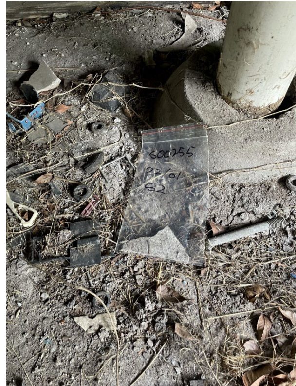
Photo 14: Potential Asbestos Containing Material (PACM) sample taken from underneath the dwelling.
