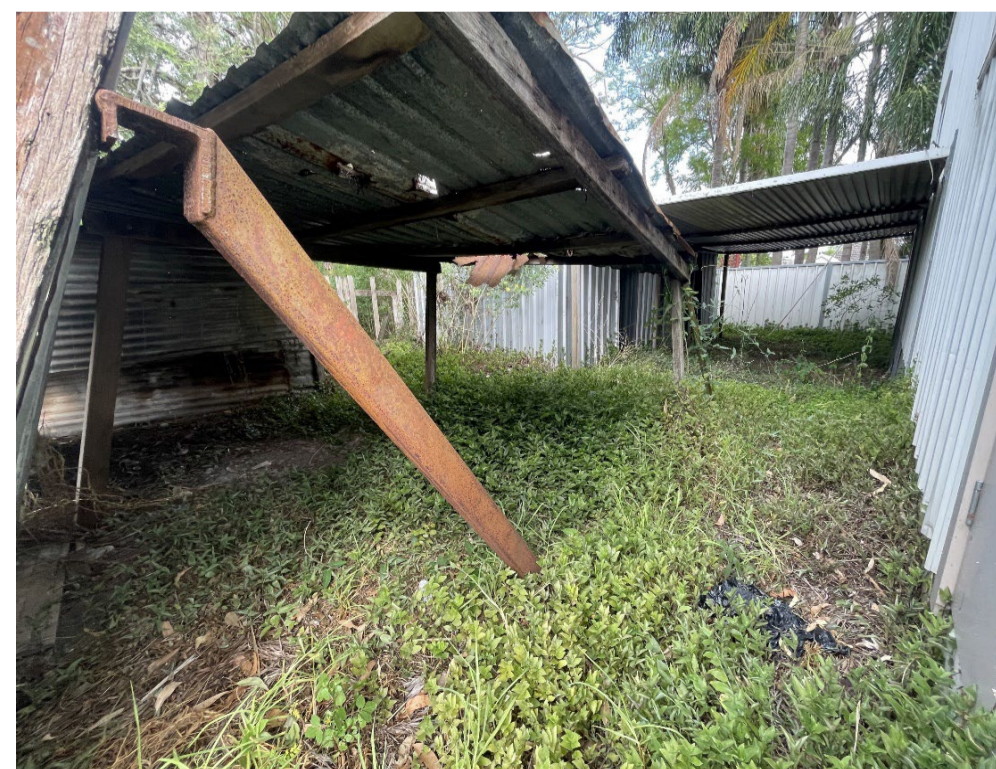
Photo 6: Overview of the small sheds adjacent to the large storage shed in the backyard.
