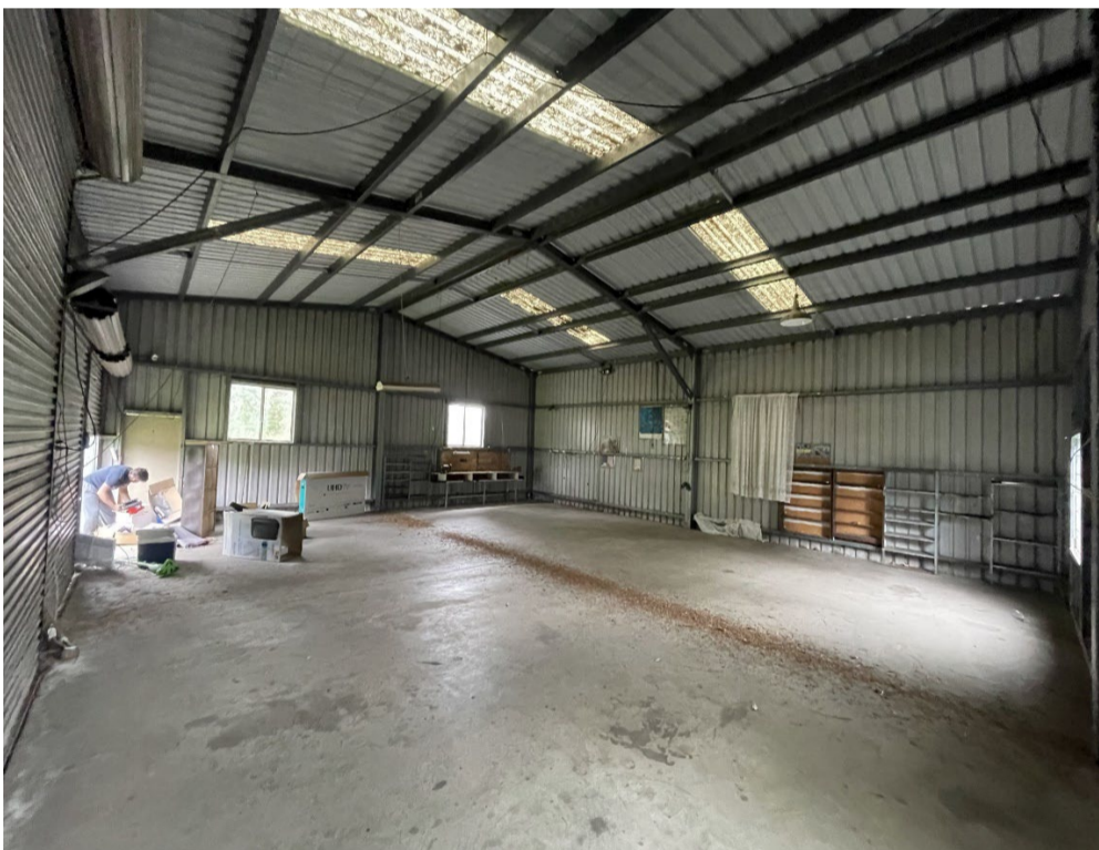
Photo 9: Internal overview of the large storage shed which is almost completely empty.
