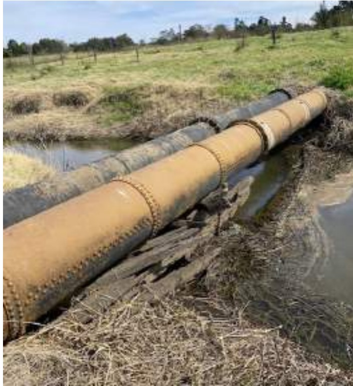
Figure 25 – Alternative view of the pipes where the timber supports appear to be rotted and failing. Source: Hunter Water.
