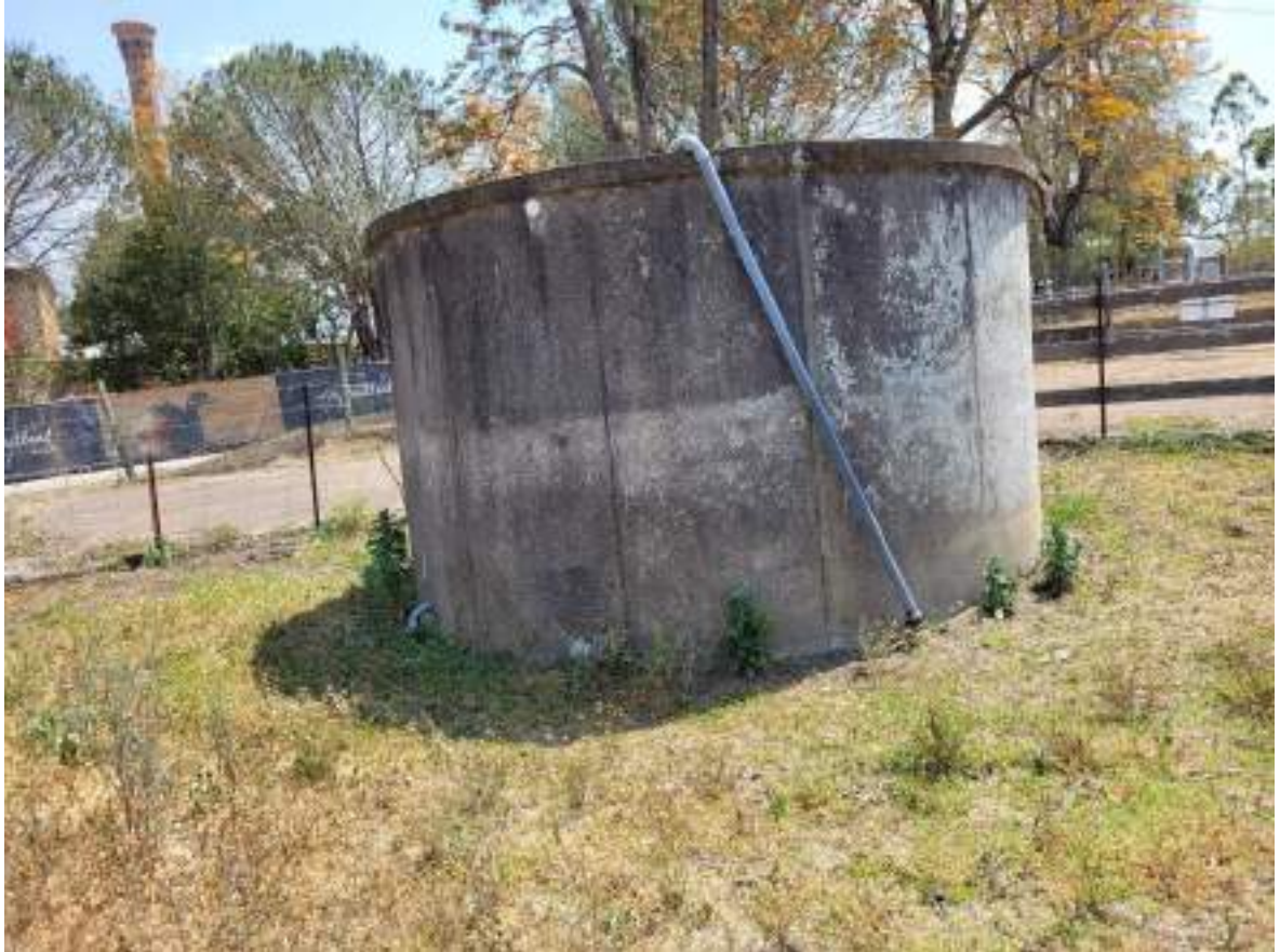
Plate 2-3. Water tank that would need to be demolished and removed. View from the east.
