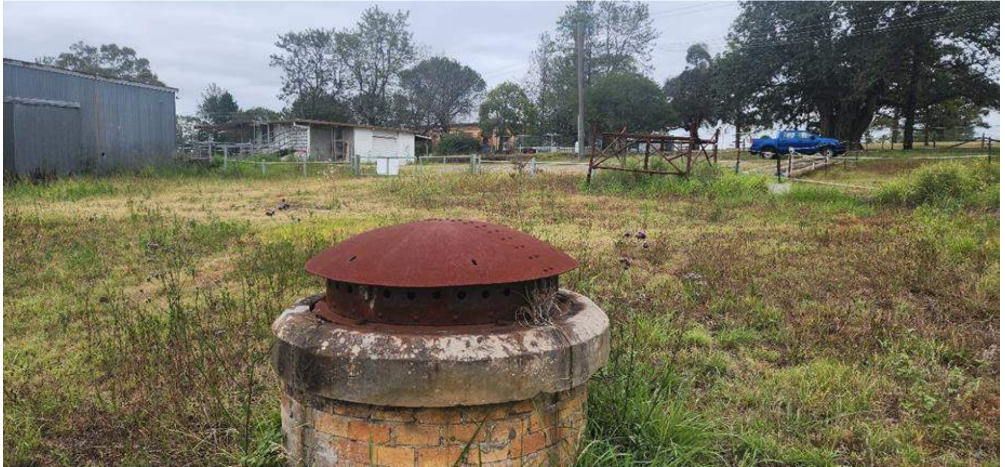
Figure 7-6. Possible air vent and/or inspection portal of former intake pipeline to Walka Water Works. Source: Eureka Heritage (2024).
