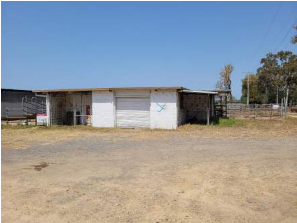
Plate 2-1. Rural shed that would need to be demolished and removed. View from the north.
