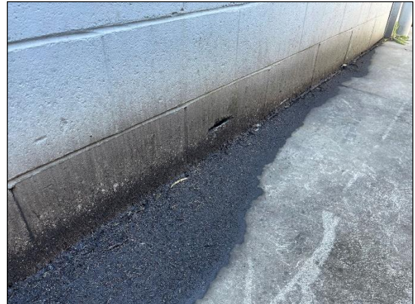
Figure 19: Staining on surface and masonry side wall of oil store
