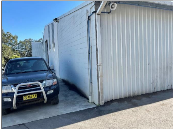
Figure 18: Staining on asphalt surface and masonry side wall of oil store
