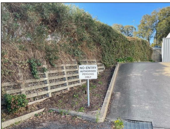
Figure 28: Retaining wall, between workshop and showroom, looking east. Backfilled with natural gravels (blue metal gravel)
