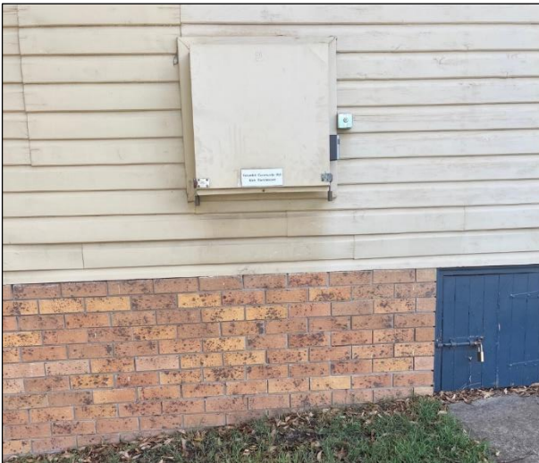
Figure 8: Switchboard on the eastern side of community centre.
