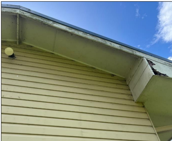
Figure 5: Damaged fibro building material on the southern side of community centre.
