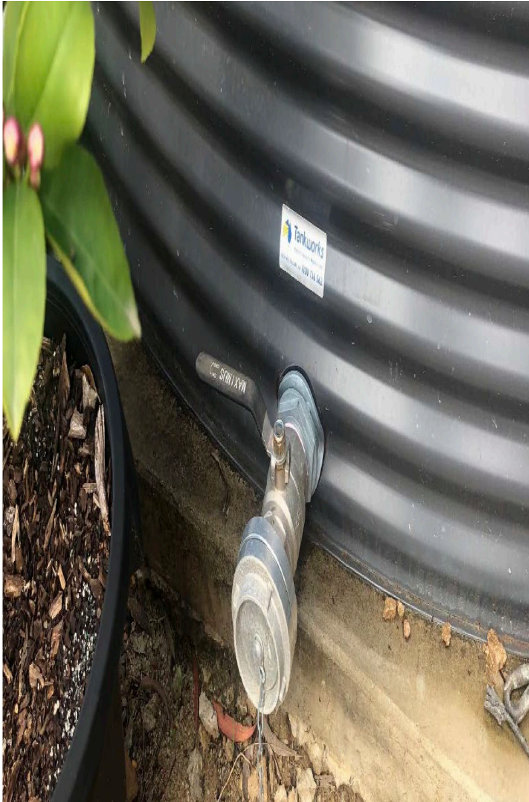
Photo 9 - 65mm Storz outlet on a non-combustible water tank.
