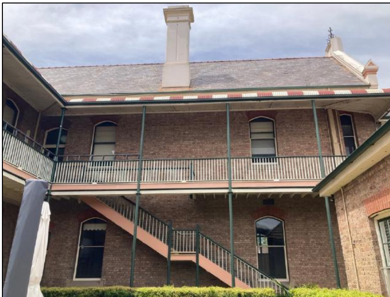
Figure 19: Southern elevation of 'Pender House' (1) showing a simple timber balustrade to the verandah.
