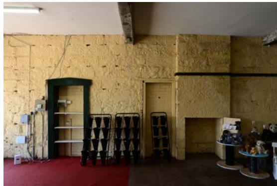
Figure 51: View of the ground floor southern side elevation showing the former window and door openings that have been bricked up, together with the former fireplace.
