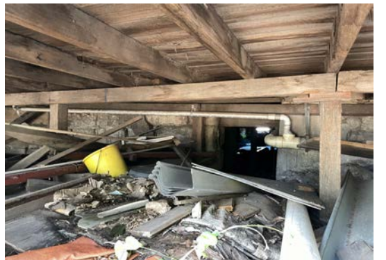
Figure 34: View of the underside to the rear loading dock and subfloor of No.101.
