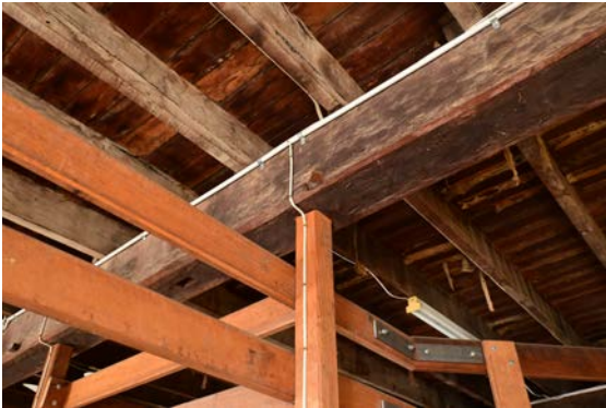
Figure 59: View of the non-original framing attaching to the underside of the original hardwood flooring and beams.
