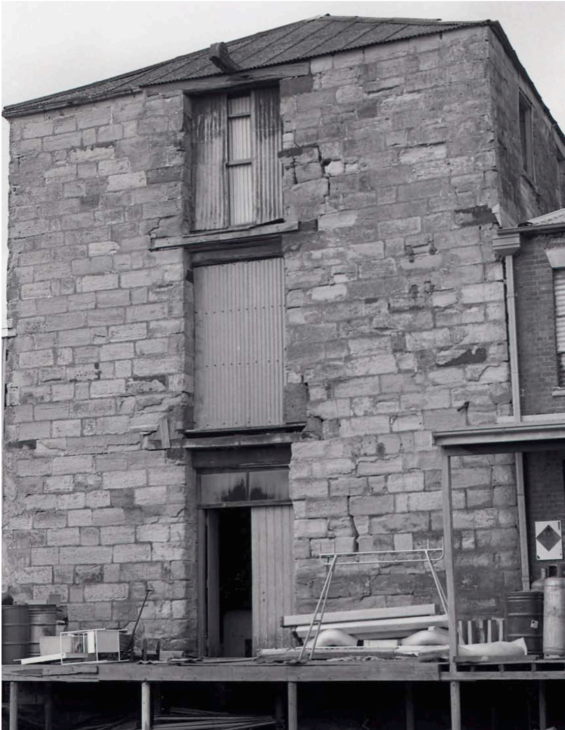
Figure 12: View of the rear elevation of the former Smiths Flour Mill, c1979. [Source: Damaris Bairstow, 1979. University of Newcastle, Living Histories C919-866]
