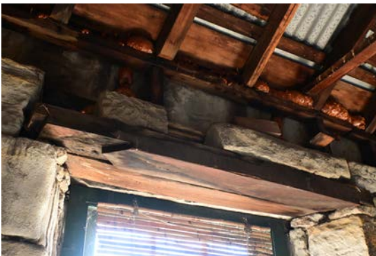
Figure 68: View of window lintel to top floor at the front.
