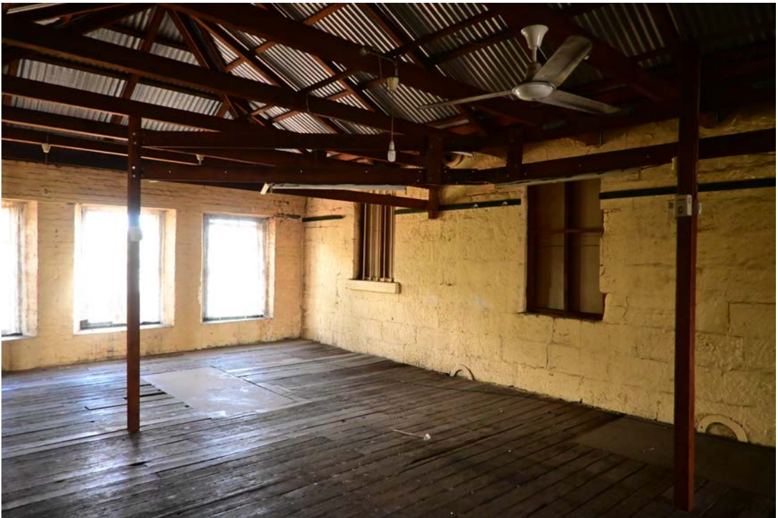
Figure 40: View of the first floor facing towards the rear and showing the former external wall to the southern side of the adjoining former flour mill.
