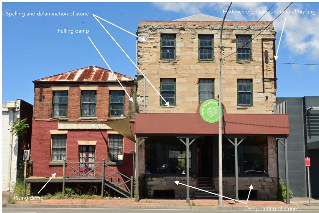
Figure 82: Visible defects to the front elevation.
