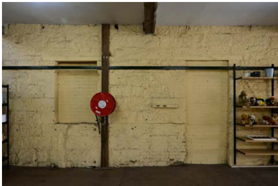
Figure 50: View of the ground floor northern side elevation showing the former window and door openings that have been bricked up.
