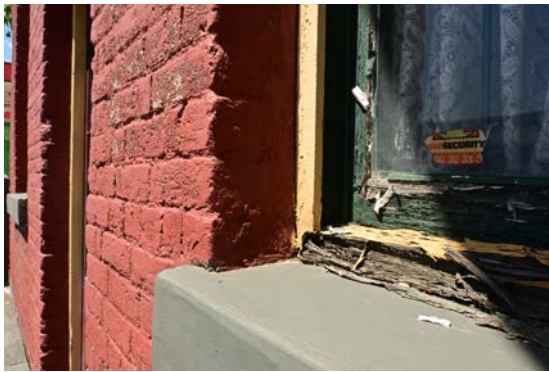
Figure 80: Visible timber rot.
