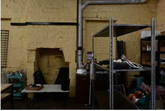
Figure 52: View of a former fireplace towards the rear of the ground floor southern elevation.
