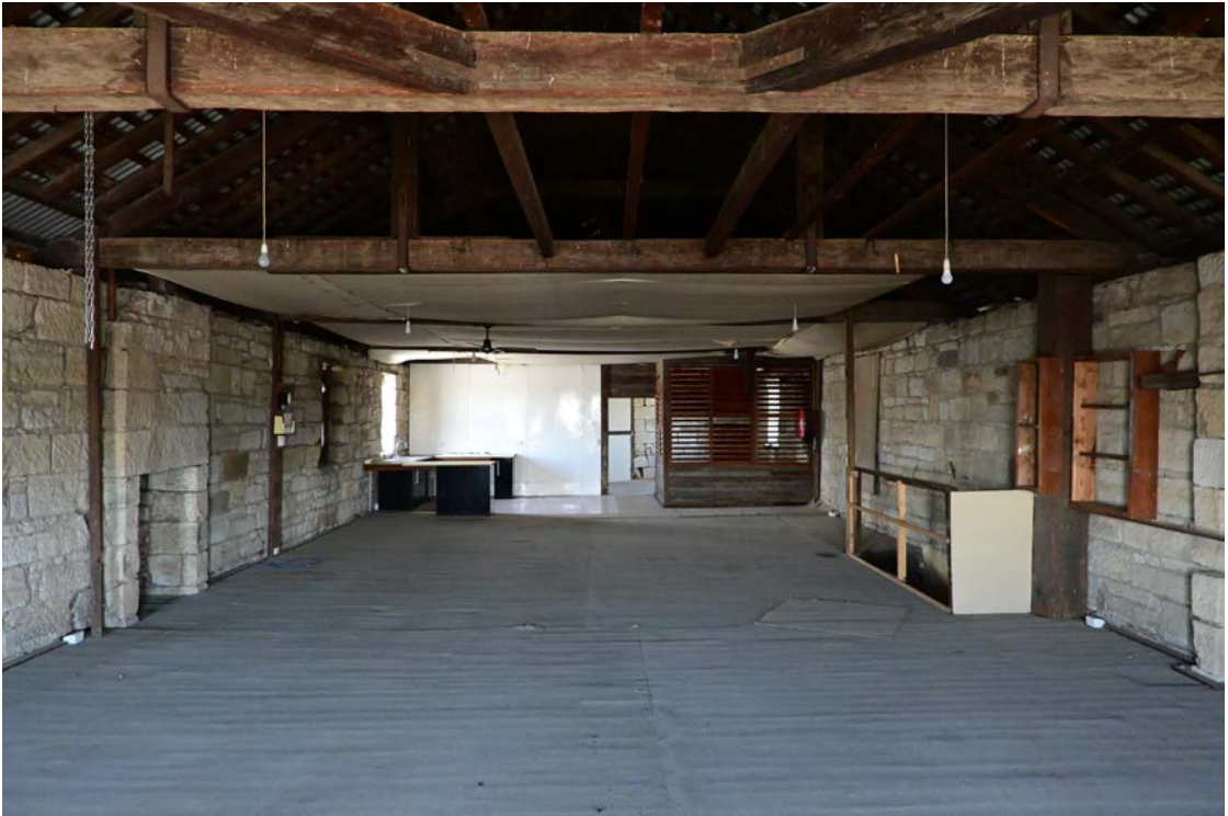
Figure 67: View of the top floor facing towards the rear and showing the studio apartment.
