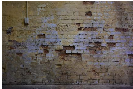
Figure 81: Visible failure to bricks.
