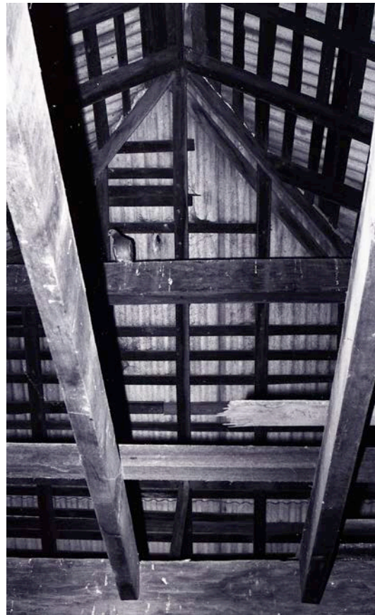
Figure 9: View of the internal roof framing to the second floor. [Source: Damaris Bairstow, The University of Newcastle, Living Histories, 2023. C919-0870]
