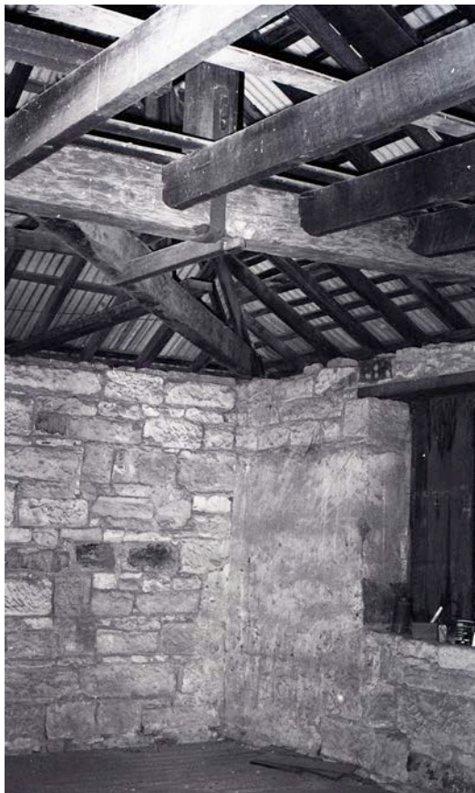
Figure 41: View of interior roof framing and walls c1979. [Source: Damaris Bairstow, The University of Newcastle, Living Histories. C919-0866]
