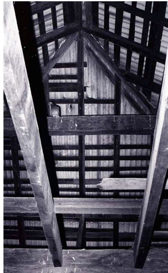
Figure 40: View of the internal roof framing to the second floor. [Source: Damaris Bairstow, The University of Newcastle, Living Histories, 2023. C919-0870]
