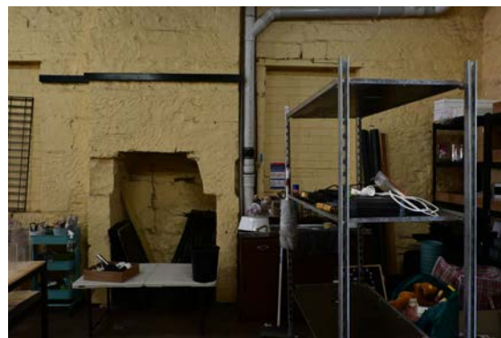
Figure 20: View of a former fireplace towards the rear of the ground floor southern elevation.
