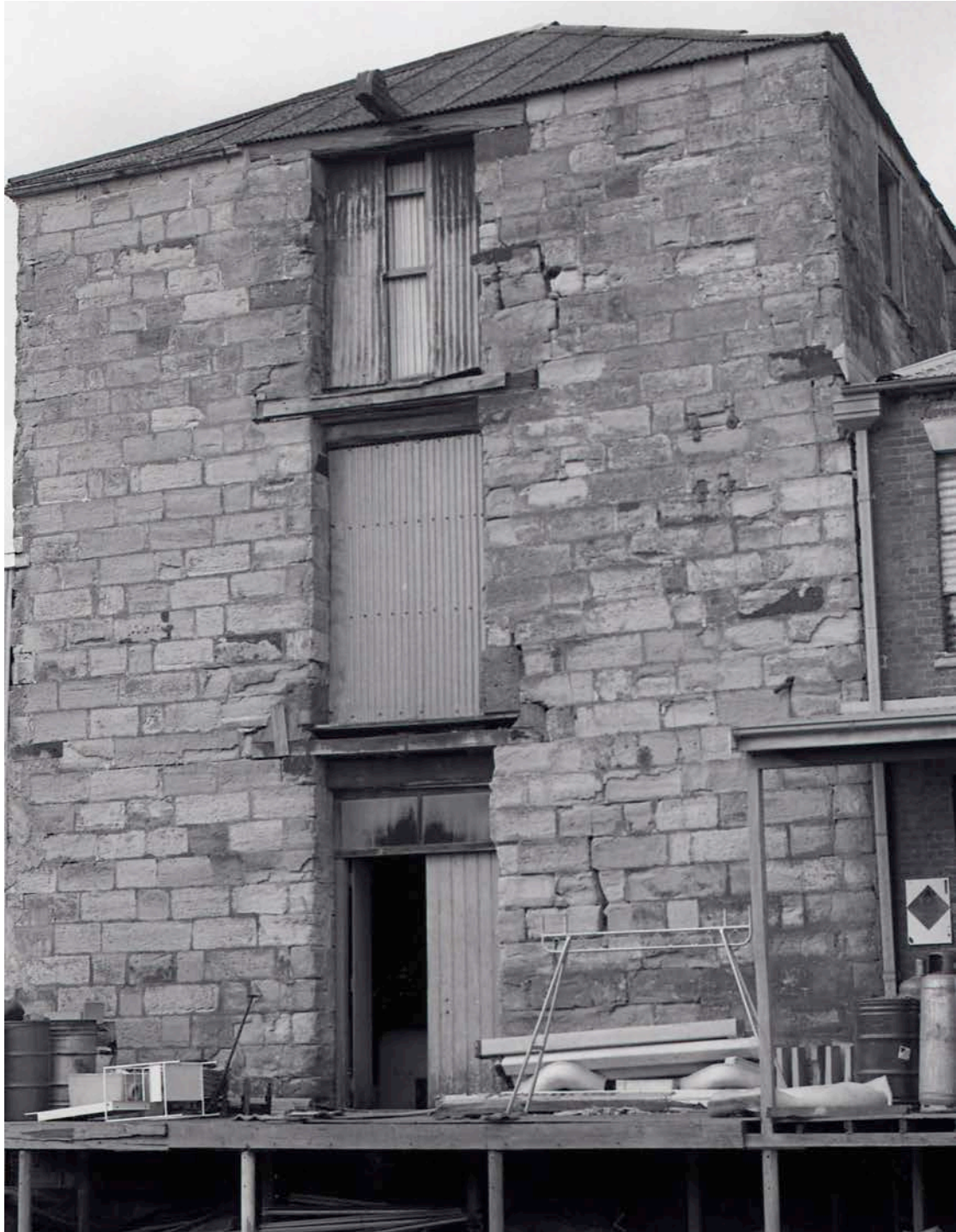
Figure 43: View of the rear elevation of the former Smiths Flour Mill, c1979. [Source: Damaris Bairstow, 1979. University of Newcastle, Living Histories C919-866]
