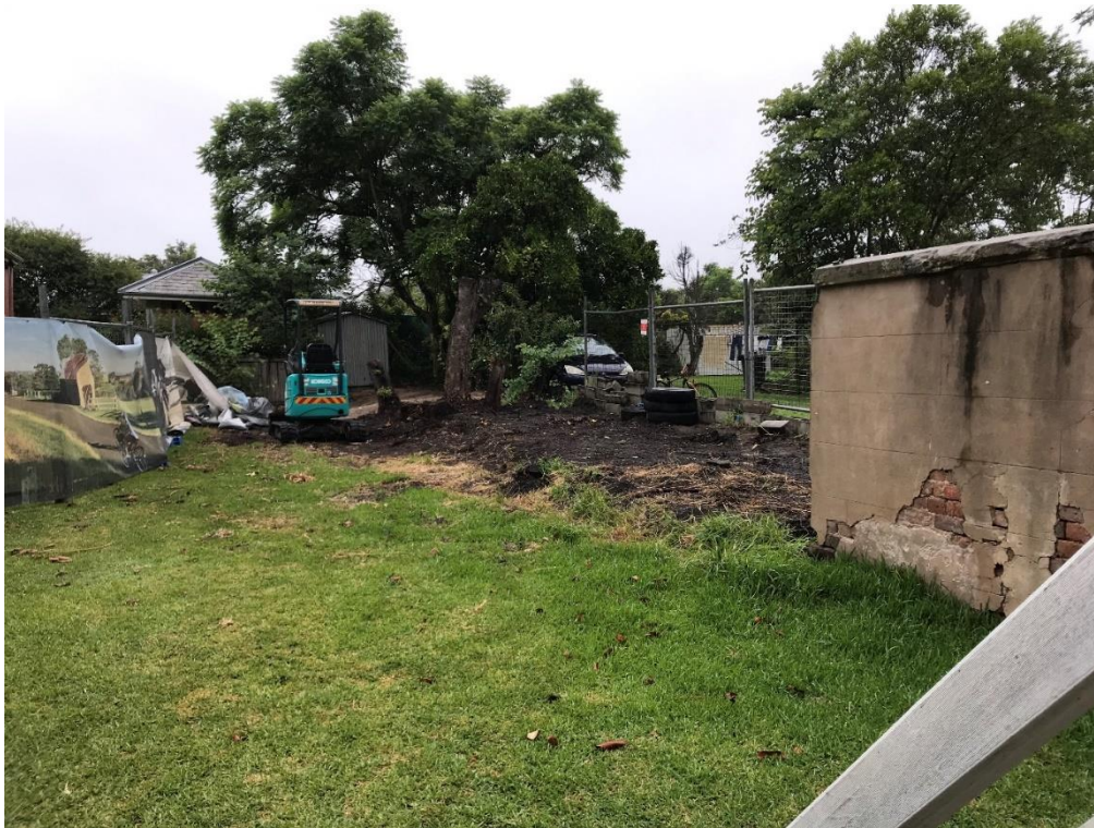
Figure 1.8 – Looking east across rear yard following demolition and removal of the timber fence. Photograph by Scott Warner, MCC.
