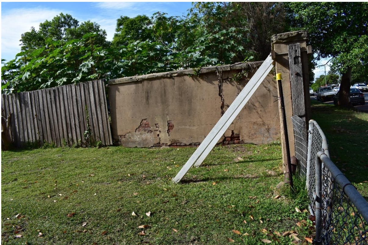
Figure 1.7 – Remnant masonry wall of rear boundary, requiring support, in March 2020. Photograph by Sue Singleton.
