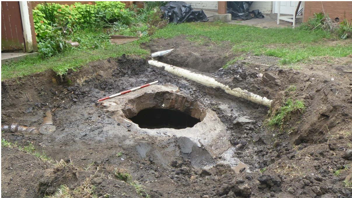
Figure 3.3 – Domed brick cover of the underground cistern located in the rear yard of the Morpeth Courthouse.
