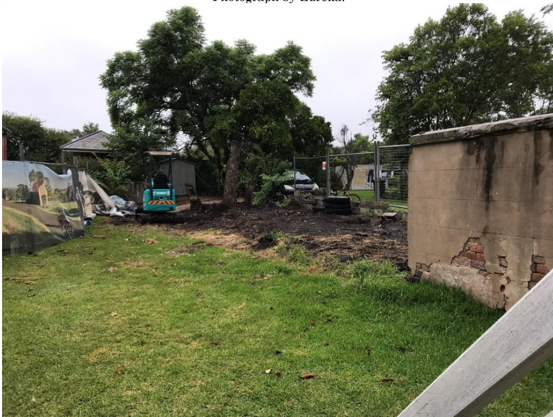
Figure 1.7 – Looking east across rear yard following demolition and removal of the timber fence. Photograph by Scott Warner, MCC.
