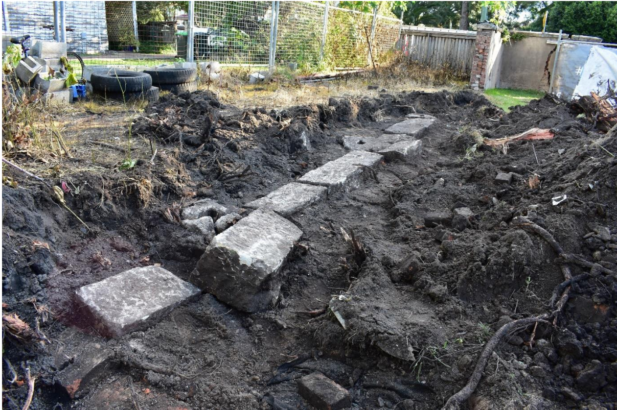
Figure 3.4 – Rear wall stable’s footings, looking south-west And surviving western masonry wall at upper right of view.
