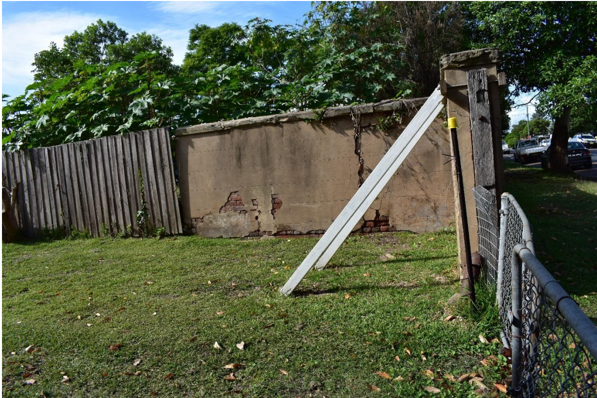
Figure 1.6 – Remnant masonry wall of rear boundary, requiring support, in March 2020. Photograph by Eureka.
