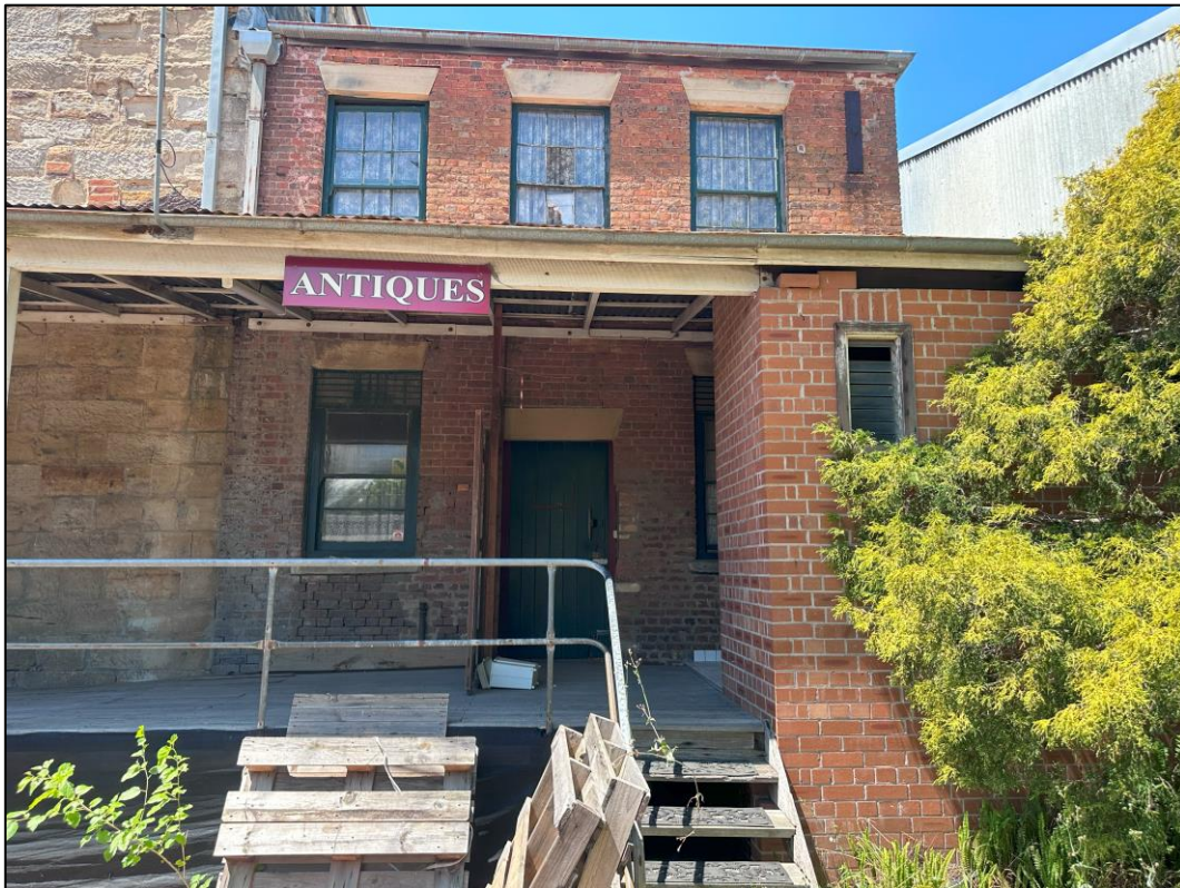
Image 6.2.2. View of the double-story brick commercial building within the northern portion of the site, as observed from the central portion of site on 10 November 2023, facing north-east.
