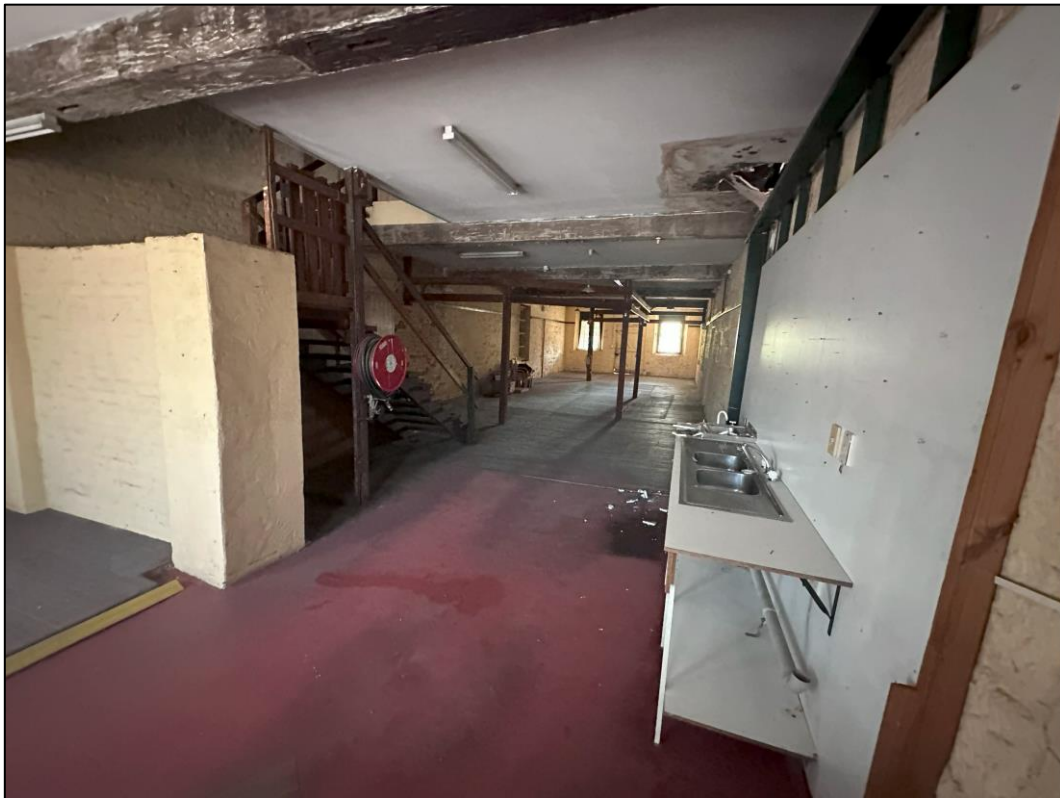
Image 6.2.8. View of first level of the double-story building, as observed from northern portion of building on 10 November 2023, facing southwest.
