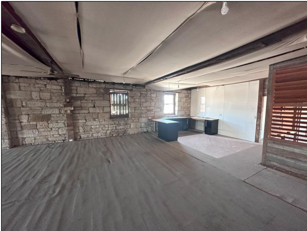
Image 6.2.6. View of third level of the three-story building, as observed from central portion of building on 10 November 2023, facing east.
