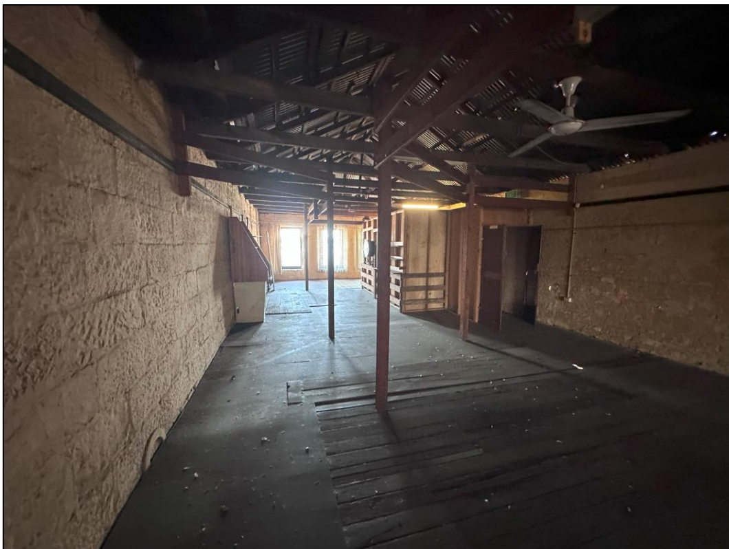
Image 6.2.7. View of second level of the double-story building, as observed from southern portion of building on 10 November 2023, facing west.
