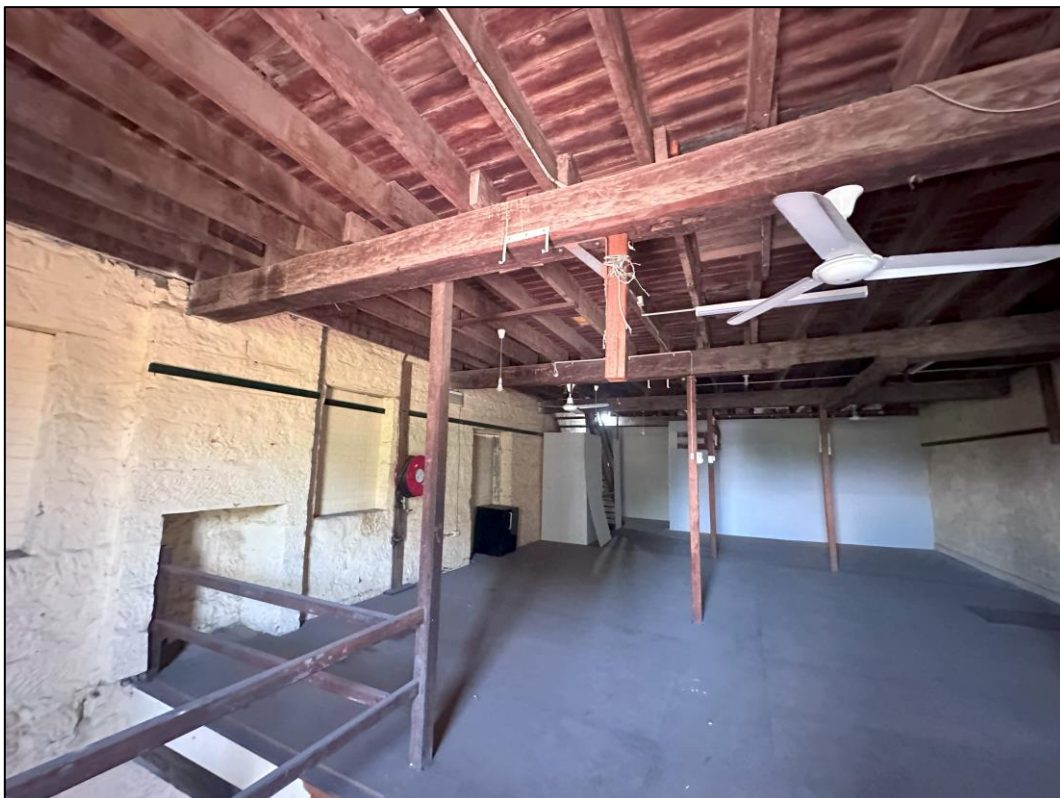
Image 6.2.5. View of second level of the three-story building, as observed from central portion of building on 10 November 2023, facing south-west.
