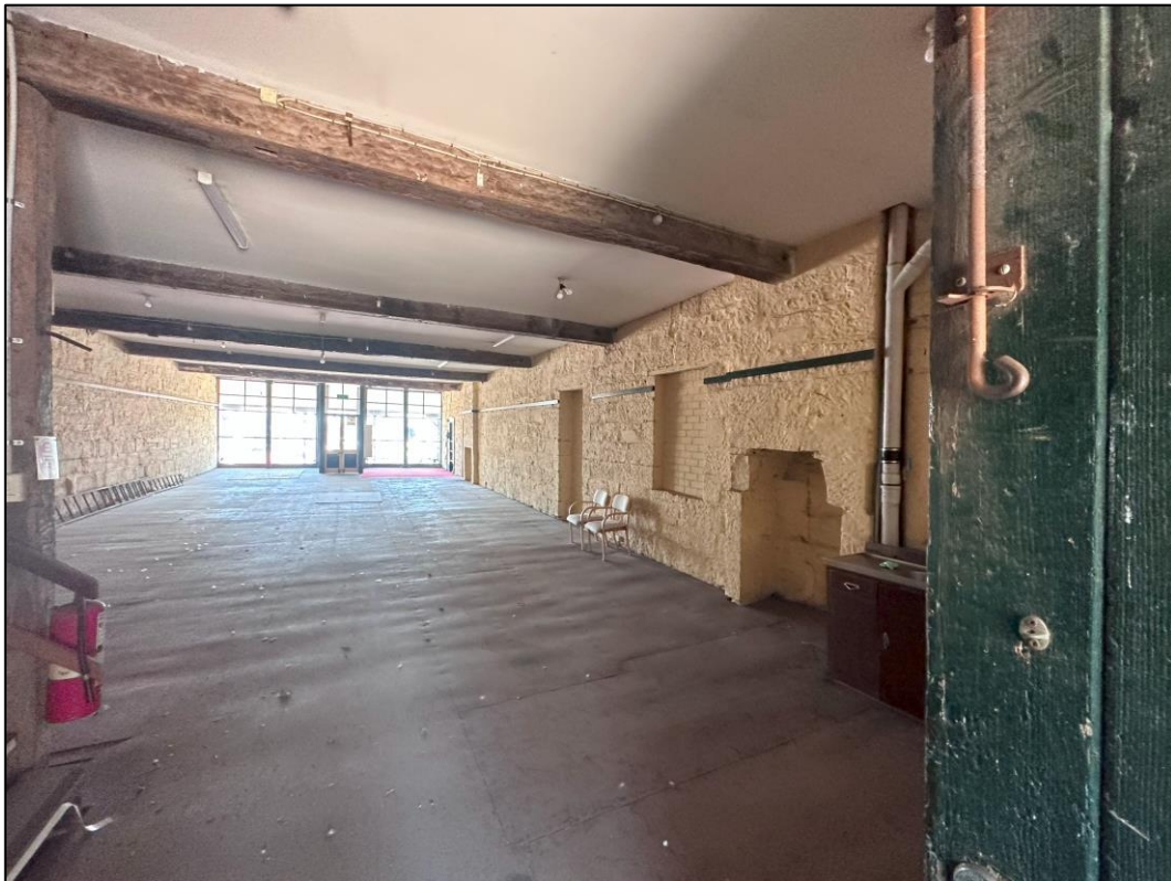
Image 6.2.4. View of first level of the three-story building, as observed from southern portion of building on 10 November 2023, facing north-east.
