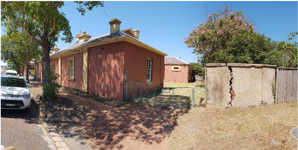
Existing vehicular crossing leading to the rear yard space off Northumberland Street
