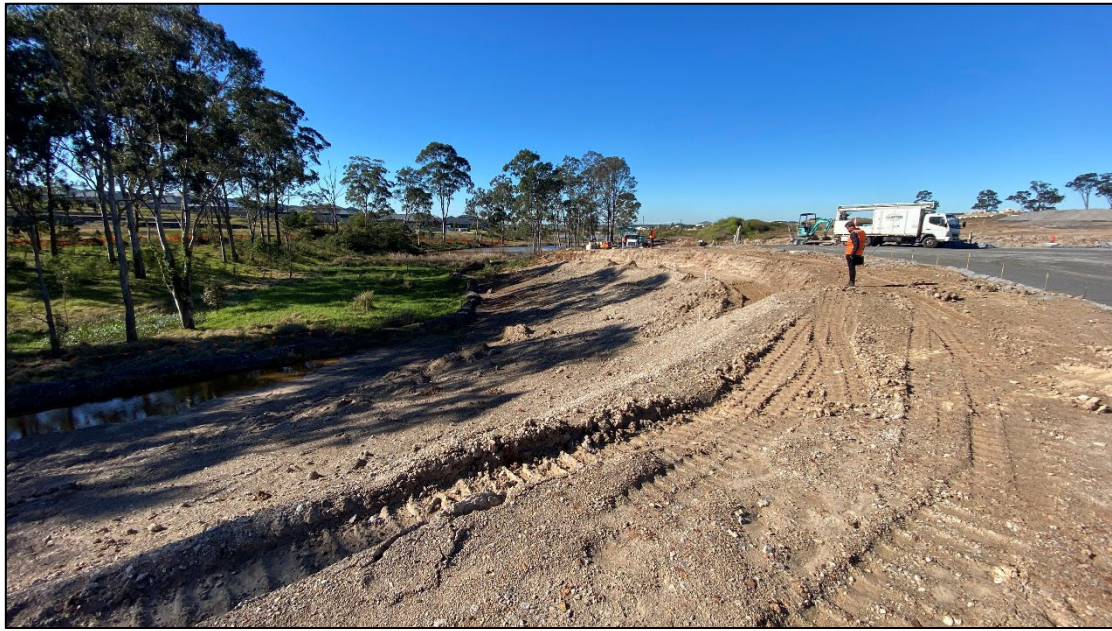
Above: Current state of construction works to the north of the proposed development. This photo shows the vegetation in the riparian area to the north that will be managed under a Vegetation Management Plan.
