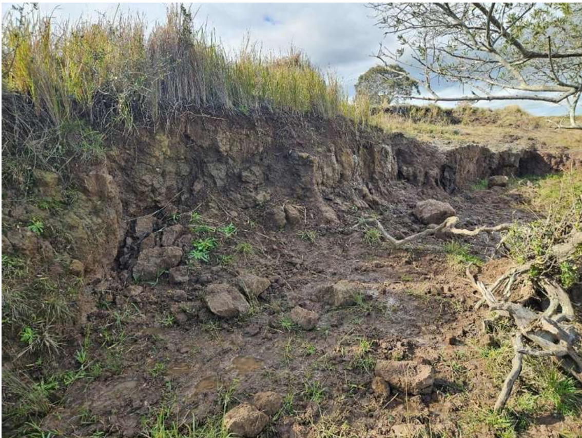
Plate 29. Erosion on the western side of Survey unit 2. (Source: Heritage Now 2024)
