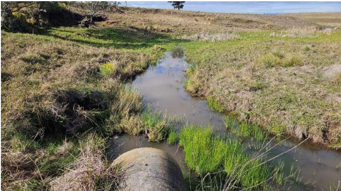
Plate 27. Water culvert for a third order creek, facing east. (Source: Heritage Now 2024)
