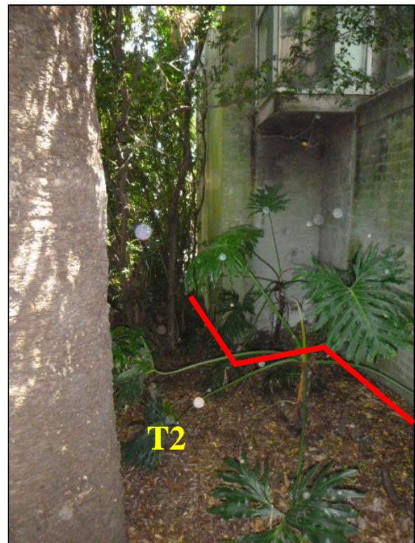
Photo 4 - Existing footings of adjacent wall to be retained to minimize impacts to roots
