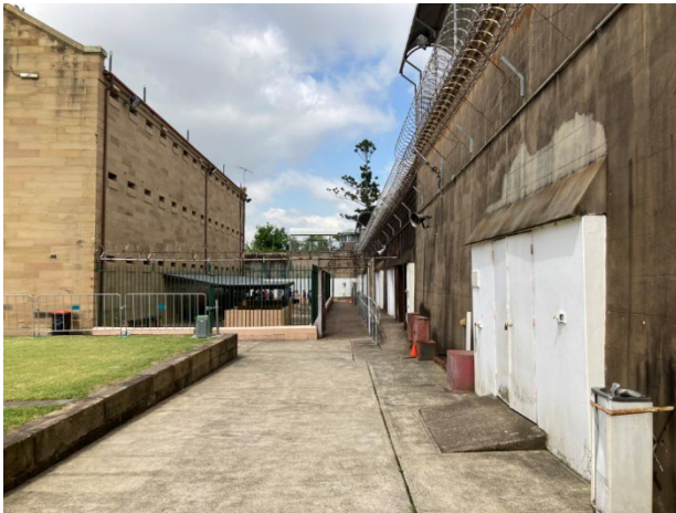
View to southwest showing 1970s addition of right, rear of B wing and concrete pathways
