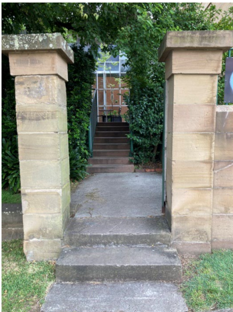
View to northeast showing entrance to café and the change in levels p to the café terrace
