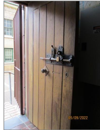
Figure 53 Typical cell door bolt and lock. This lock is one of the more recent Abloy Lock types.
