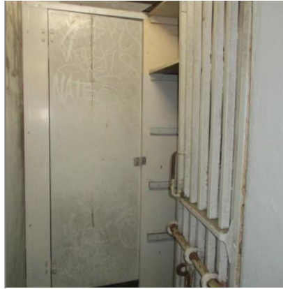
Figure 22 View from inside a typical A Wing cell without a grille door. There is no rebate in the reveal. This opening was created at the time of doubling the cell numbers.
