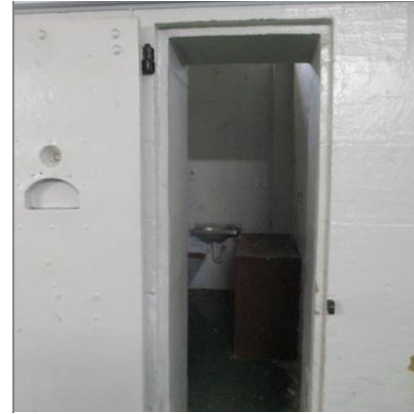
Figure 23 View from inside a typical A Wing cell with a grille door and a solid door. There is a rebate to house the grille door in the closed position.
