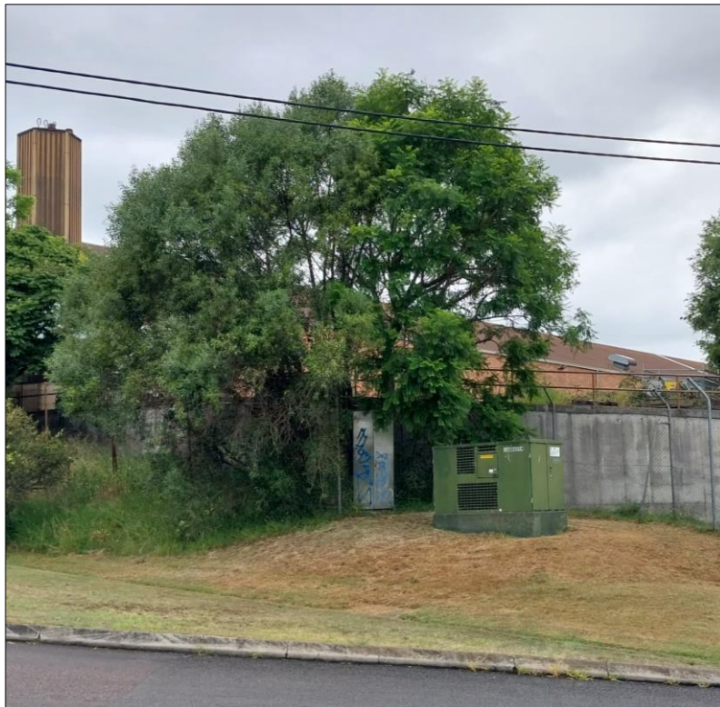
Figure 15 View of Asset Building 14 from corner of Cumberland and Lindsay Street (looking southwest). Source: Barr Planning 2023
