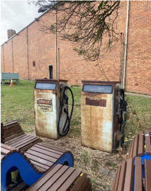
Photograph 1 – Existing Fuel bowsers (standard & super) onsite, vent pipes visible to the rear wall
