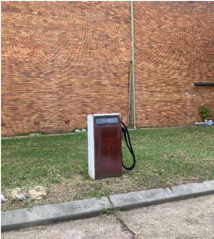
Photograph 2 – Existing Diesel Fuel bowser onsite, vent pipes visible to the rear wall
