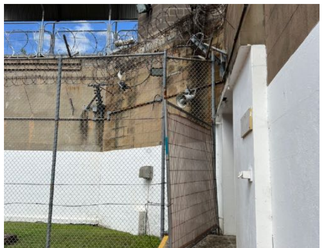
Figure 39 Concrete framed portal entrance to the Reception Store as viewed from the internal courtyard. source: Heritas, 2022.
