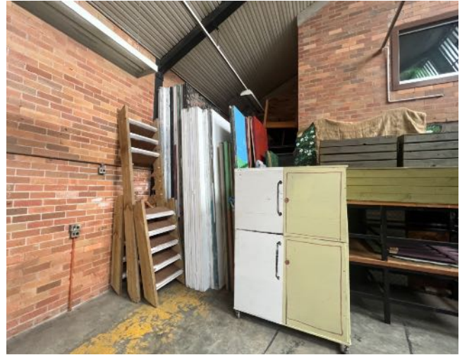
Figure 41 View of exposed brickwork to interior of Saddlery with timber lined raked ceiling. source: Heritas, 2022.
