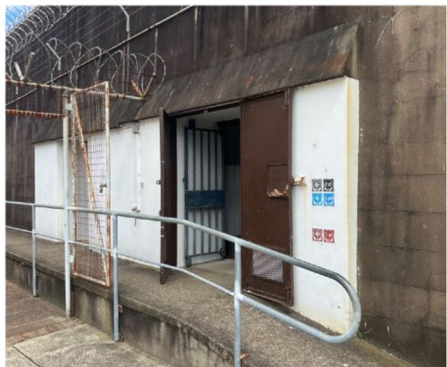
Figure 51 Concrete framed portal entrance with heavy metal security doors to perimeter wall of Gaol. source: Heritas, 2022.
