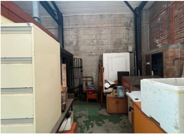
Figure 34 Internal view of Reception Store with exposed trusses, brick walls and concrete blockwork. source: Heritas, 2022.
