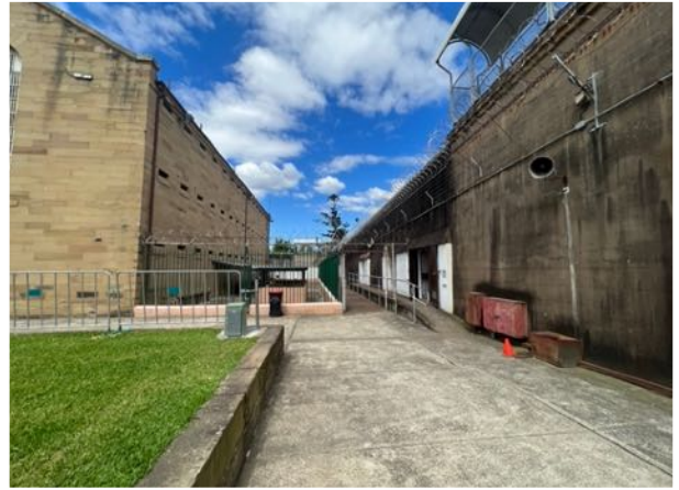
Figure 19 View looking south-west towards the rear of 'B' Wing. Ramp to 1970s addition at right with concrete pathways to surrounds. source: Heritas, 2022.
