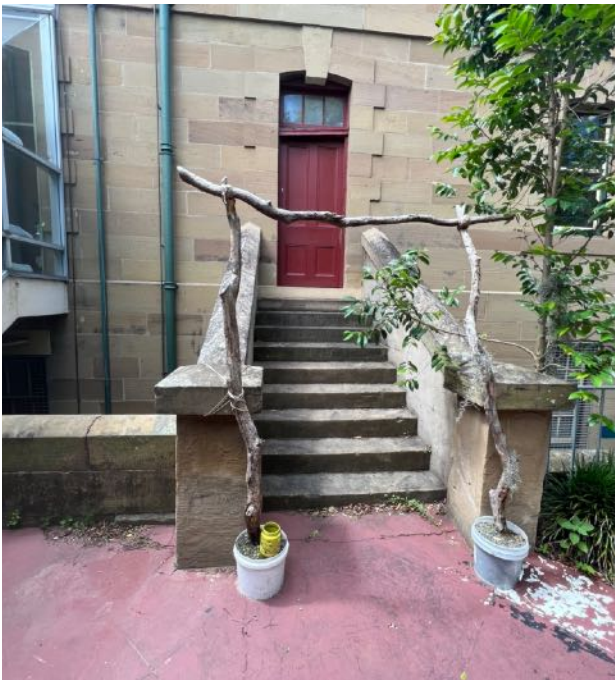
Figure 60 Entrance to the Lieutenant Governor's Residence from the existing café terrace. Timber framed door with triple paned highlight window. Simple keystone and quoining detail to door surrounds. source: Heritas, 2022.
