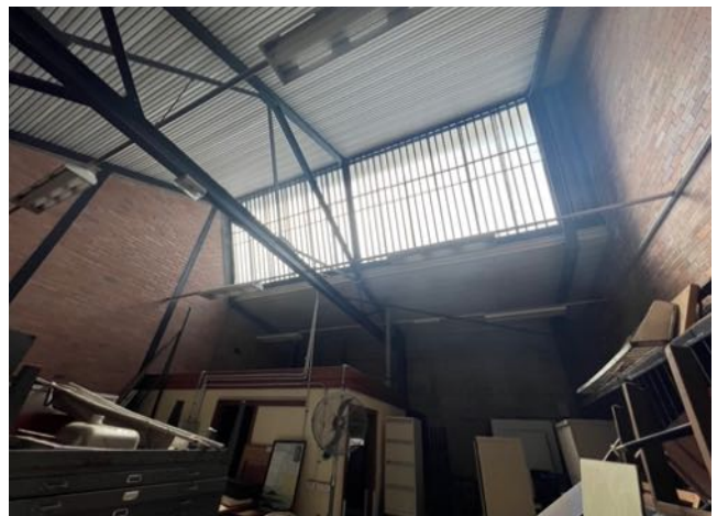
Figure 37 View of clerestory windows with metal security grille over the Reception Store. source: Heritas, 2022.
