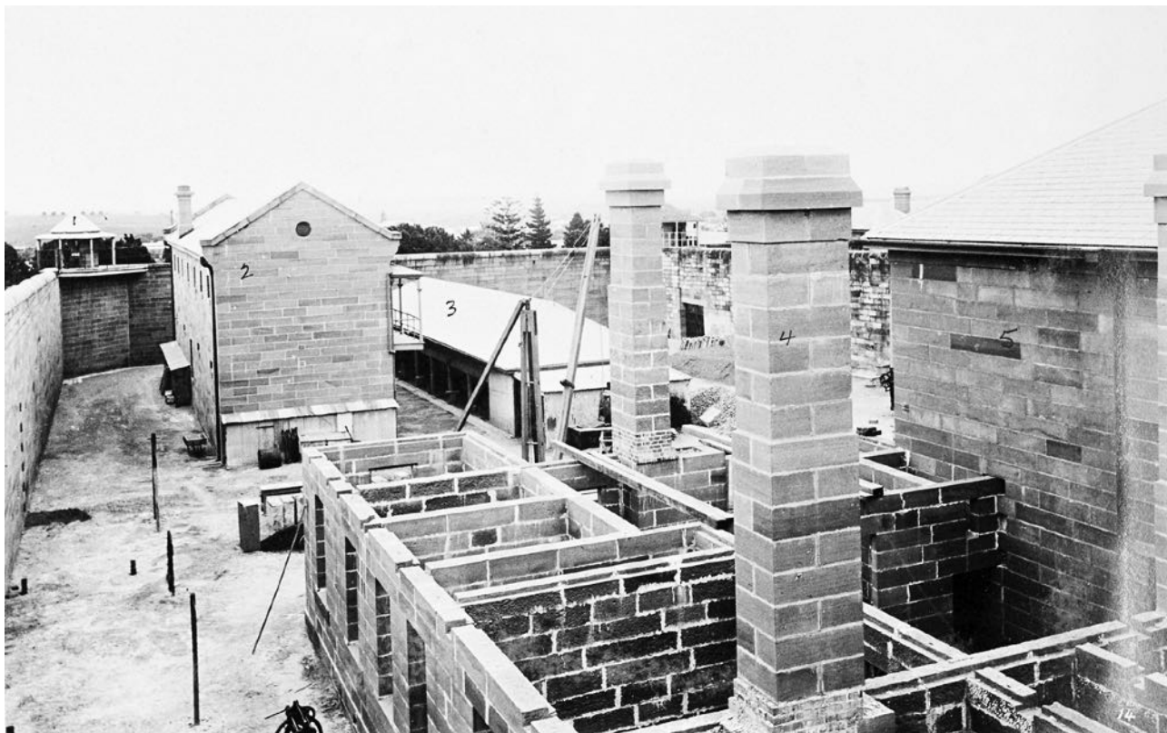
Figure 19 The Eastern Extension, construction of new female cell wing in foreground, c1897. source: Photographic views of NSW Prisons DOCS.
