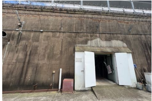
Figure 33 Internal opening to perimeter wall providing access to the former Laundry space within the Store building. source: Heritas, 2022.
