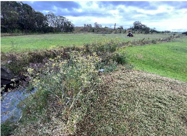
Figure 12 Stormwater outlet to the former market garden site. source: Heritas, 2023.
