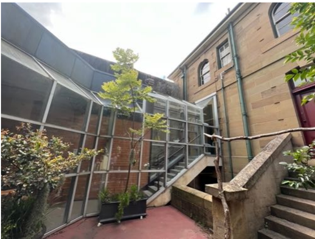
Figure 33 Glazed linkage (1980s extension) adjoining the northern façade of the former Lieutenant Governor’s quarters. Modified window opening with entry to late 20th century amenities. source: Heritas, 2023.
