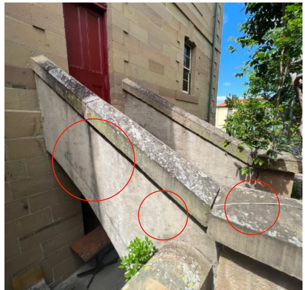
Figure 36 Rendered masonry stairwell with ashlar coursing and saddleback coping. Areas of cracking outlined in red. Evidence of original exposed stonework to pillar at right. source: Heritas, 2023.
