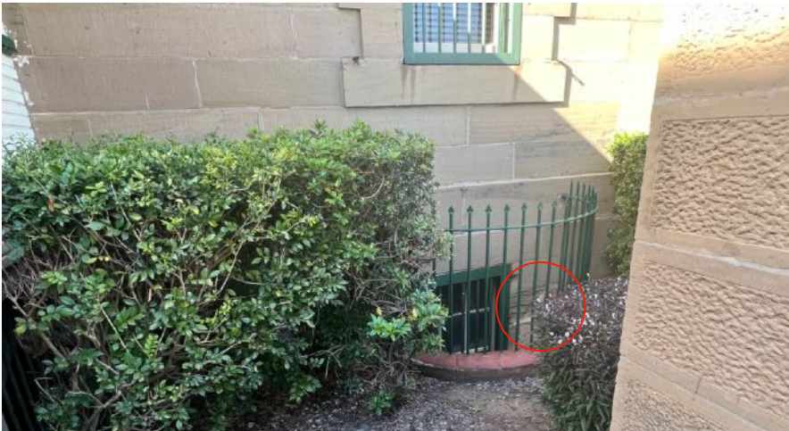
Figure 49 Metal spear head palisade fencing to surrounds of basement level windows. Note delamination of stone at right of window. source: Heritas, 2023.
