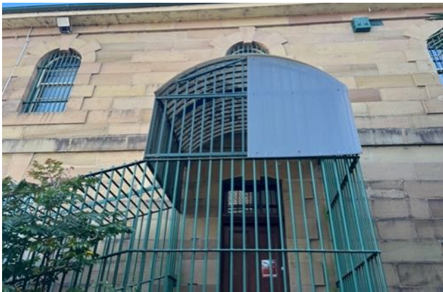
Figure 39 Detailed view of security cage over southern entrance with metal bars and Corflute sheeting. source: Heritas, 2023.
