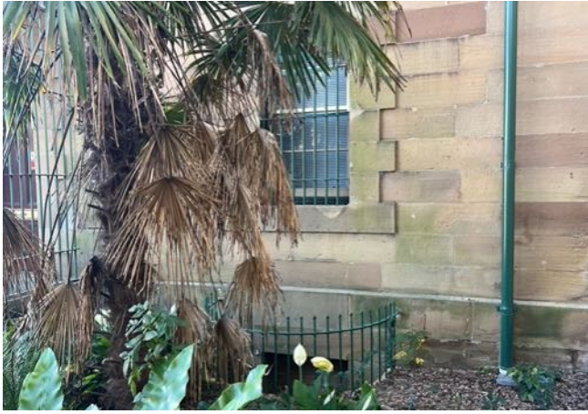
Figure 37 View of southern façade with quoined windows and metal security grilles. Spearhead palisade fence to surrounds of former basement window opening (infilled with brickwork). source: Heritas, 2023.
