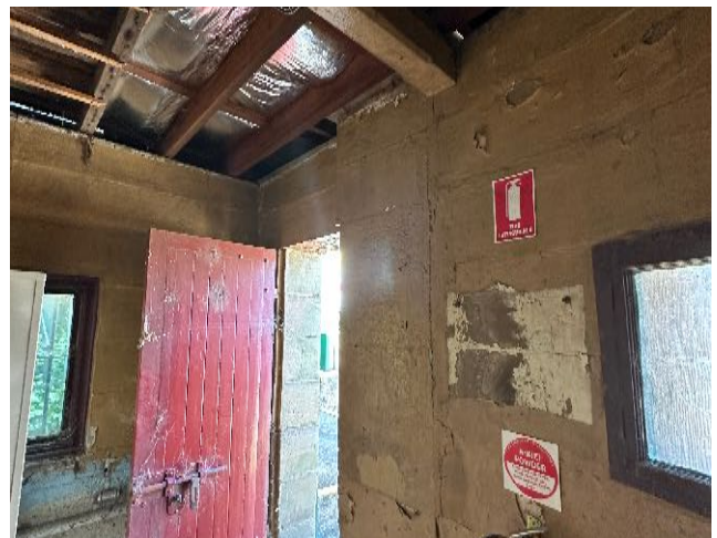
Figure 55 Interior of Sentry Box with painted sandstone and timber framed windows. source: Heritas, 2023.
