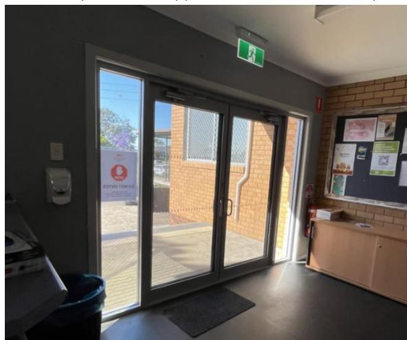
Figure 18: Non-compliant Full Height Glazing
