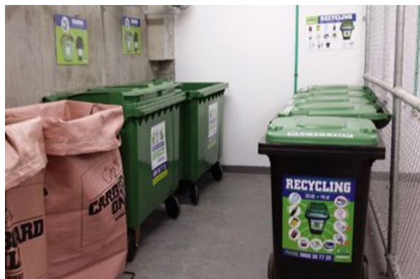
Figure 3-137 Waste and recycling areas should allow for sufficient space to manoeuvre bins and sort waste for recycling
