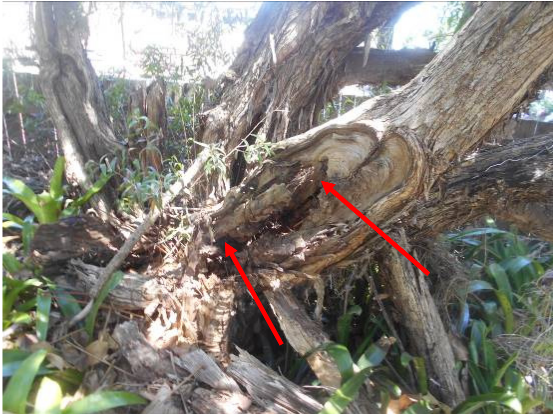
Figure 11 – showing the location of Tree 12. Tree 12 has extensive decay in the trunk at ground level
