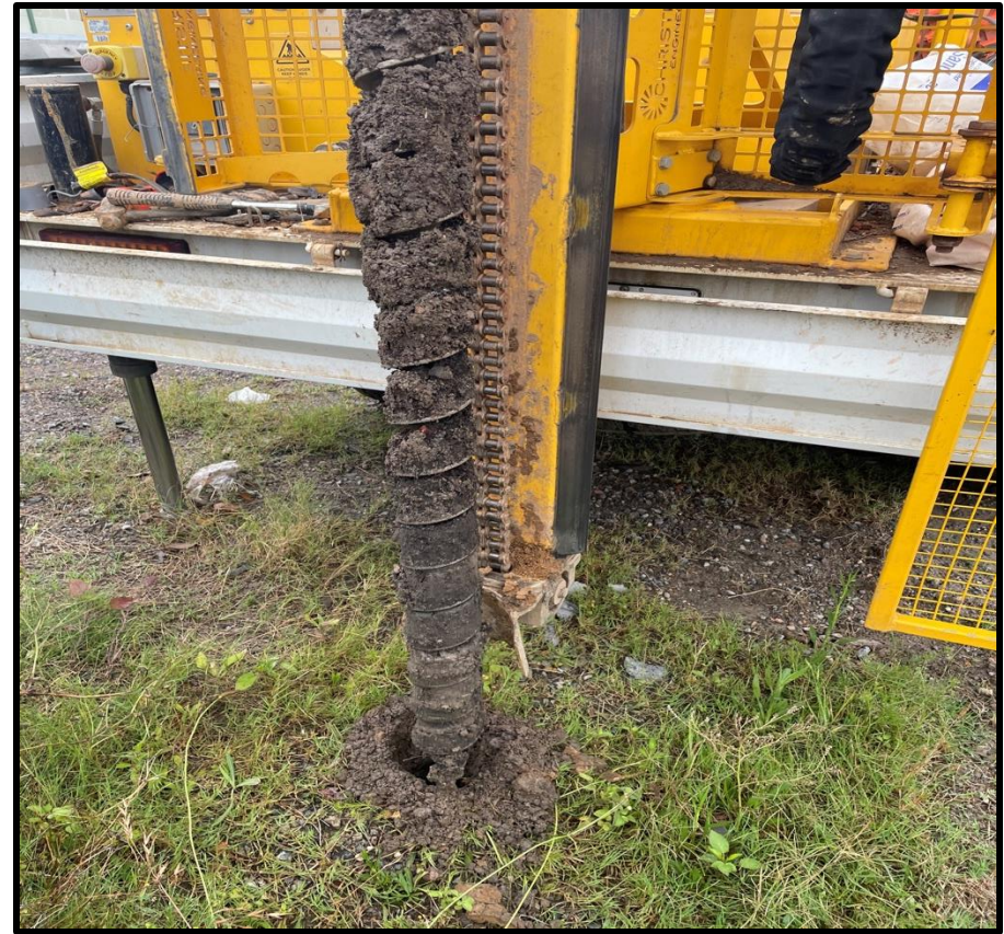
Figure 27. Sandy gravelly clay identified in BH3.
