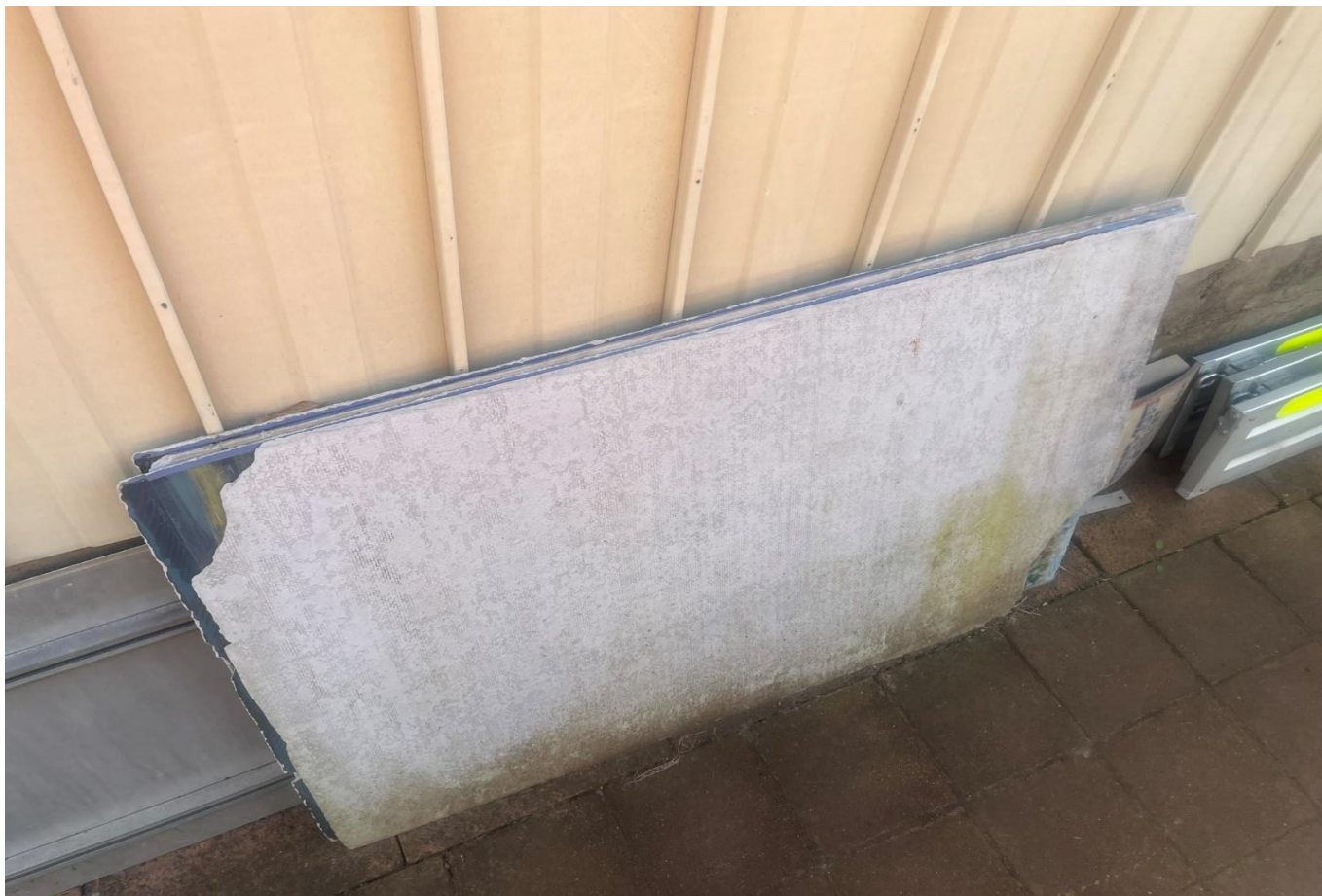
Photograph 15 - Showing stored PACM observed on the southern side of Dwelling 2.
