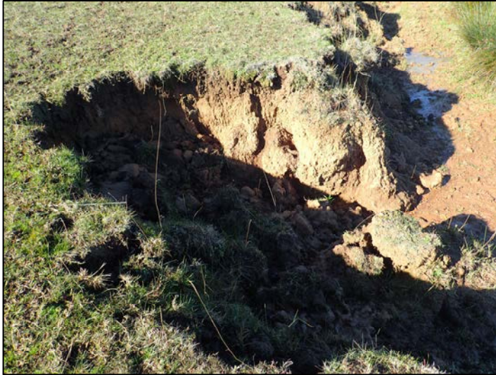
Figure 6.17 Eastern side of the creek, northern end showing creek bank collapse
