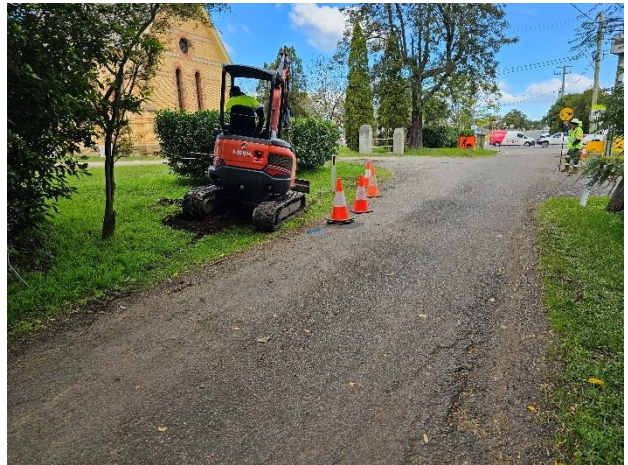
Photograph 6: Facing south from approximately 6m northwest of BHQ05. Excavator at borehole location (BHQ05). New England Highway in background.
