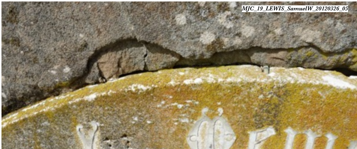
The marble inscription panel for Samuel W. LEWIS (#19, 1903) has held in place despite deterioration of the surrounding sandstone edges. Thomas Browne secured the panel with additional copper staples.
