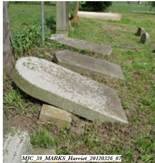
The forward lean of the Harriet MARKS base (#39, 1869) reveals that it was leaning significantly forward before it fractured and fell.
