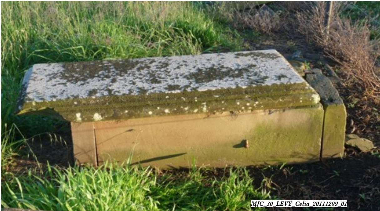
Movement of the top slab, coupled with rusting of the fixing cramps, is placing the Celia LEVY boxtomb (#30, 1854) at risk of collapse.
