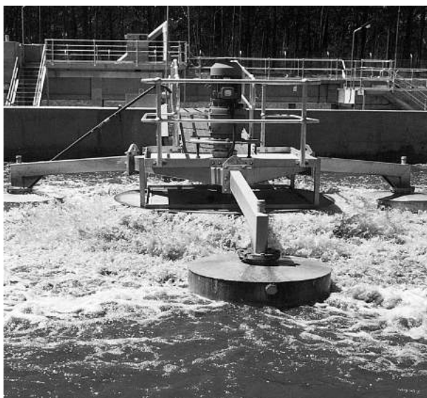
Biological treatment: air is pumped through the wastewater providing oxygen to micro-organisms as they break down the waste.
