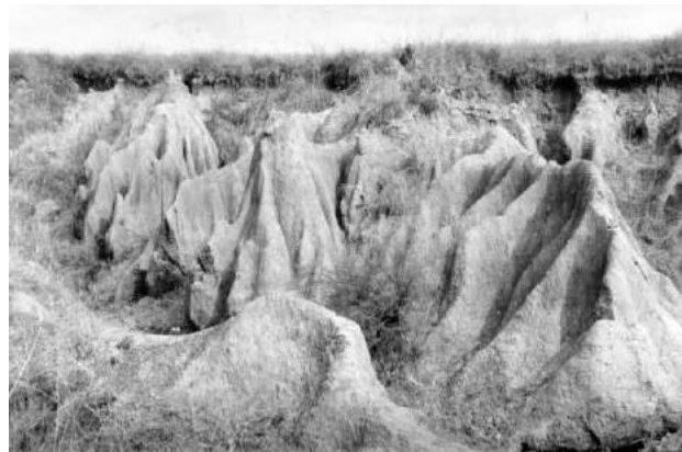
An example of severe gully erosion. Once established this type of erosion is extremely difficult to restore.
