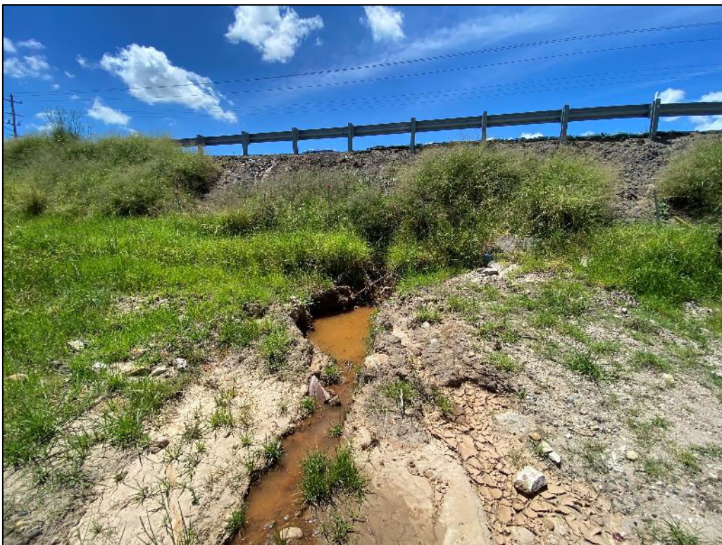
Plate 5: Looking east towards Cessnock Road showing water seepage and erosion.
