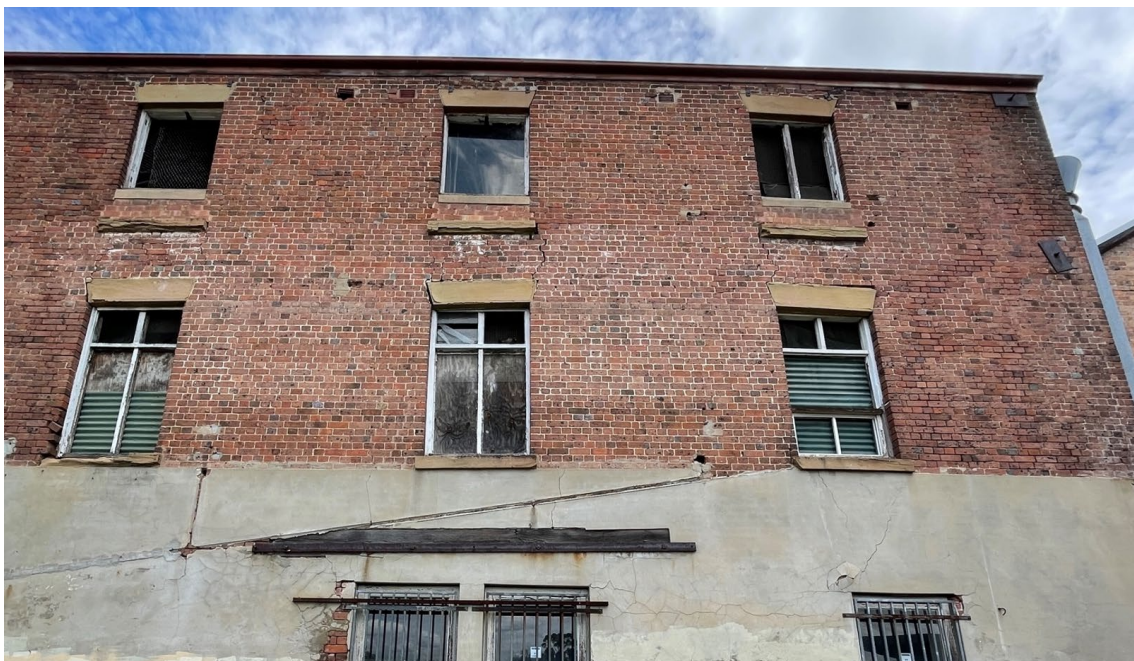
Figure 11 – External View of the Distorted Lintels & Cracked North Wall
