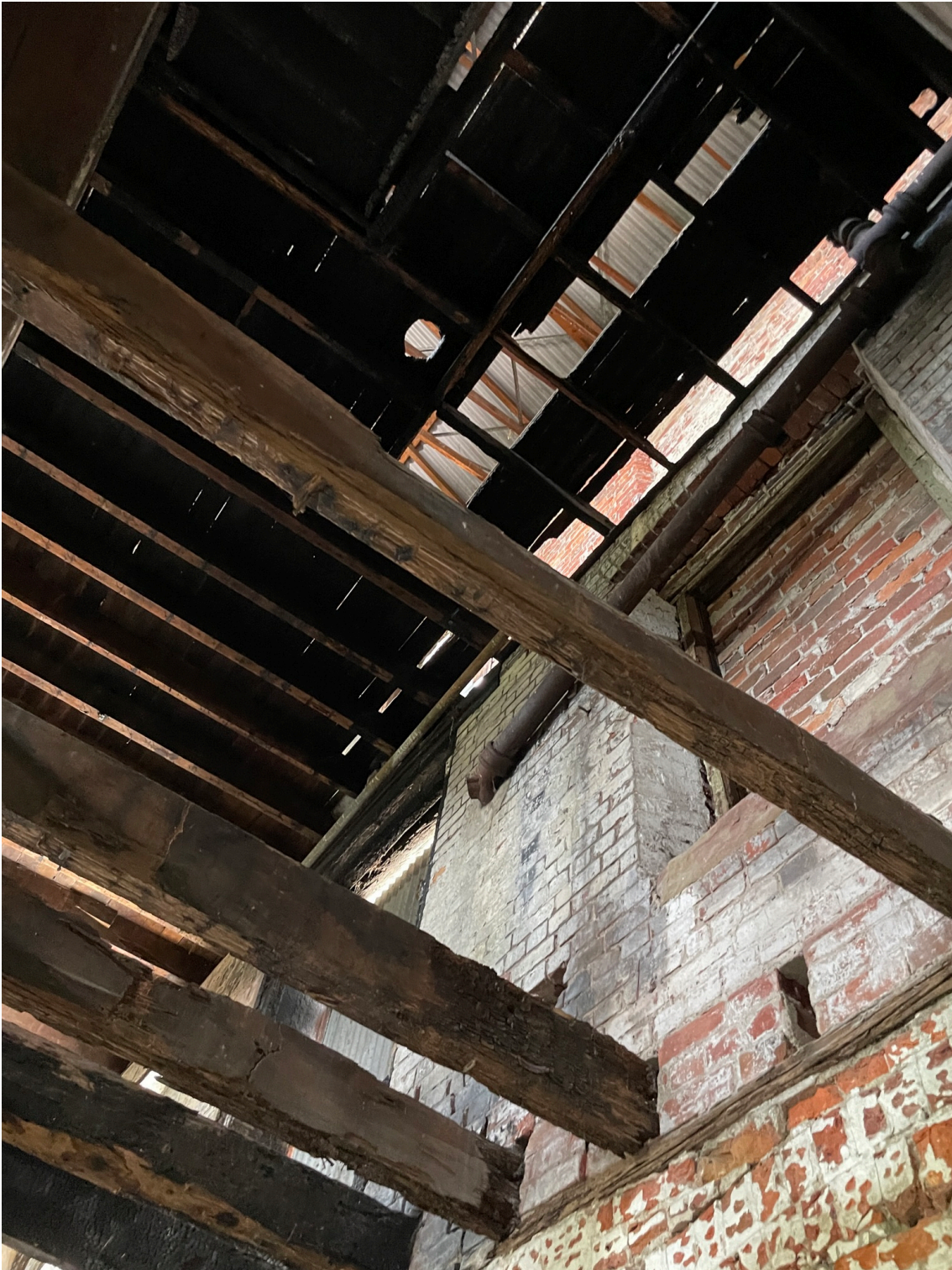
Figure 9 – Internal View of the Fire Damage to the First & Second Floor Timber Framing
