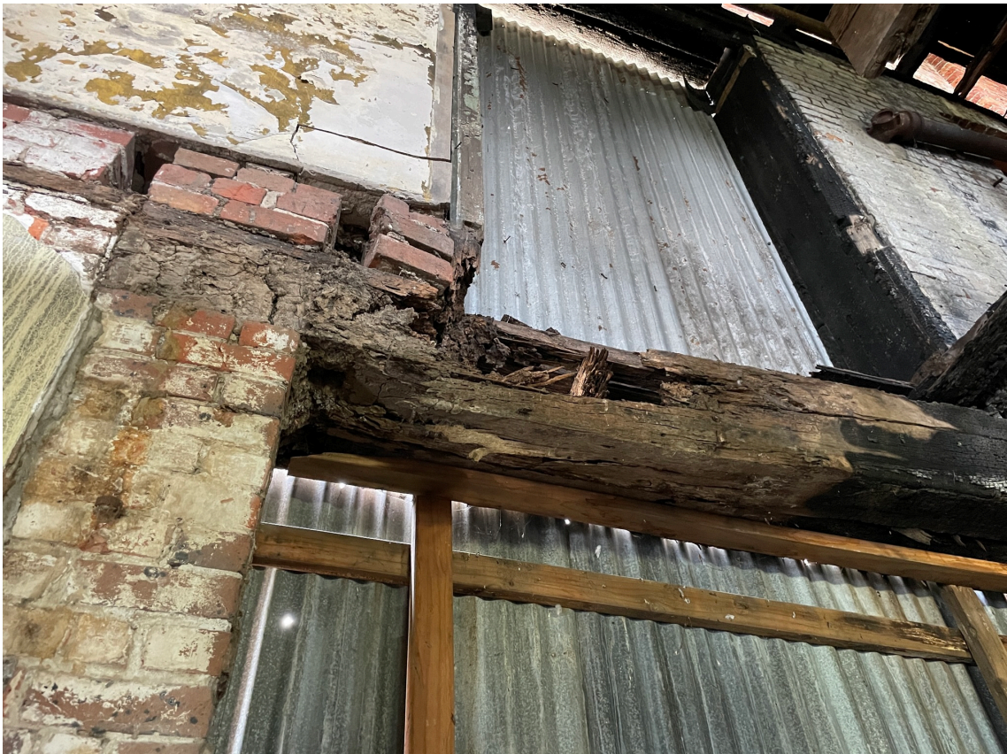
Figure 8 – Internal View of the Fire Damage & Rotted Timber Lintel
