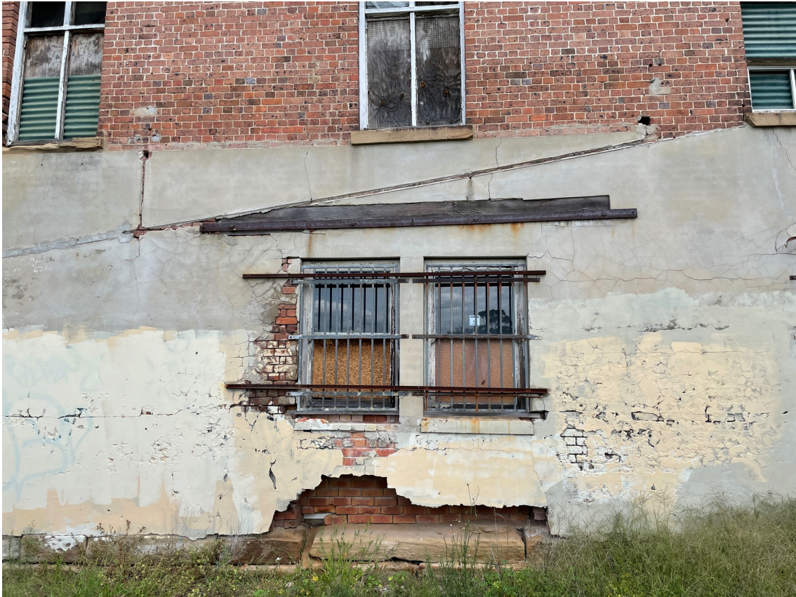
Figure 10 – External View of the Partially Collapsed North Wall
