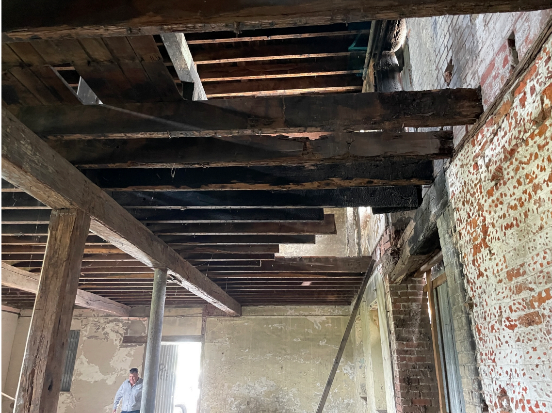
Figure 7 – Internal View of the Fire Damage to the first Floor Timber Framing
