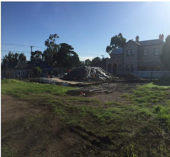
Photograph 3: Looking north east at stockpile area, covered in black plastic, stockpile on building footing
