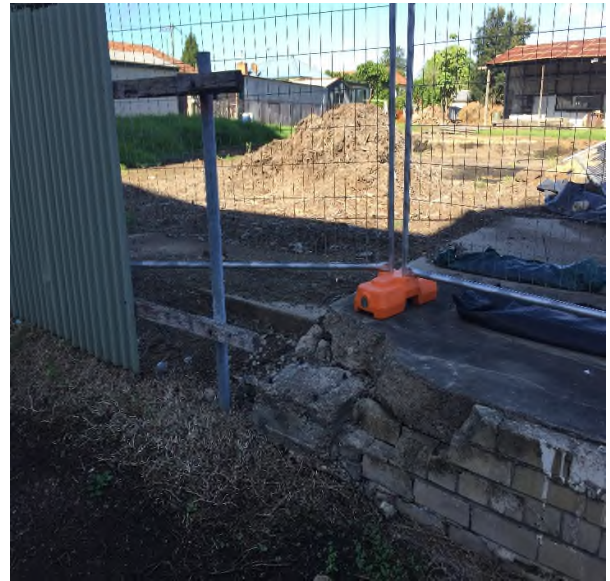
Photograph 2: Gap in silt barriers on eastern boundary of site
