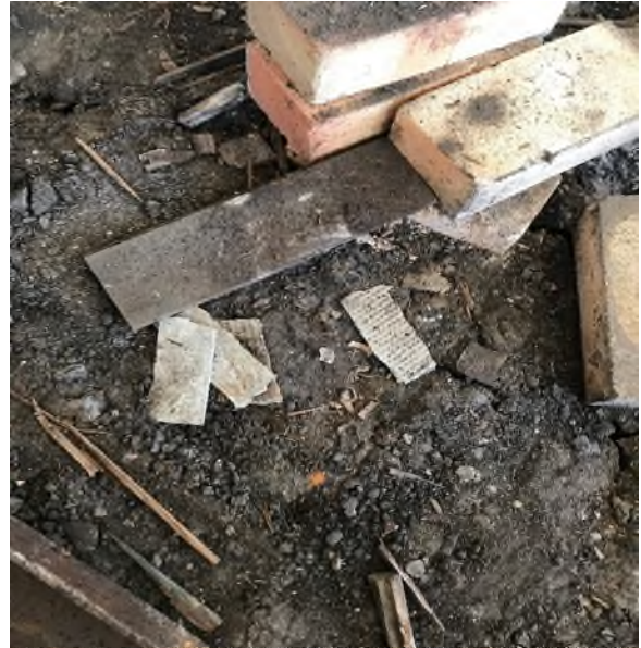
Photograph 26: Showing ACM within the remaining structure on northern boundary of the site. ACM seen within brick footings.
