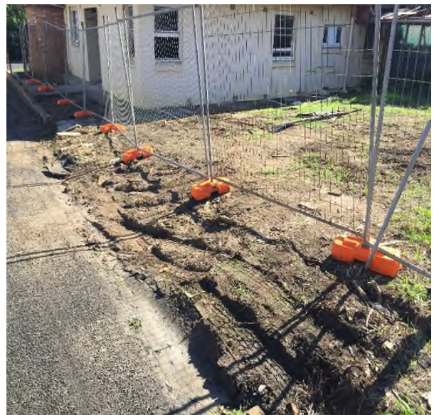
Photograph 20: Showing western boundary of the site, showing no silt barriers
