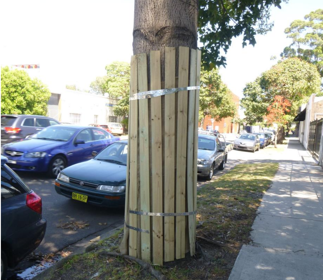
Figure 11 – Example of acceptable Trunk Protection batten installation
