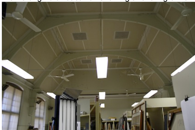
View toward north-west wall with original ceiling and dormer windows concealed behind Plasterboard
