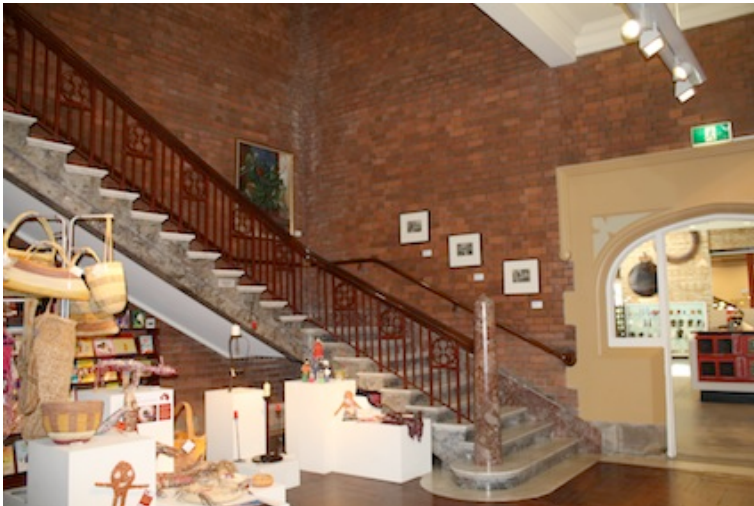
View of north corner of Stair Hall showing pink marble newell post. Note evidence of former water entry in north west corner.
