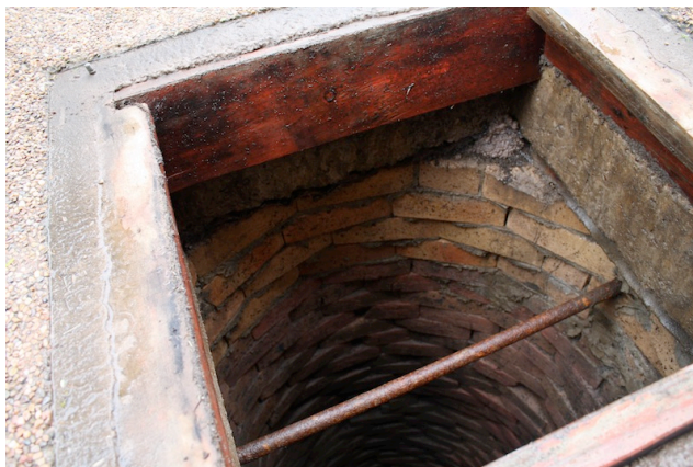
View of the well with the steel plate cover removed located to the south-east of the Rear Building
