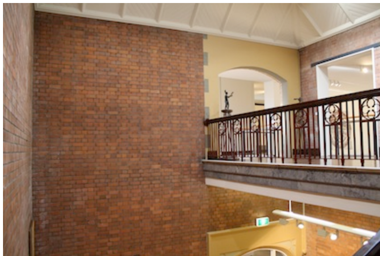
View toward north-east wall showing new opening on south-east wall with new building beyond.
