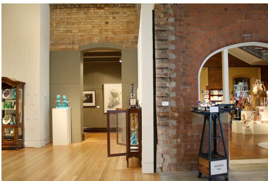
North-east facade of the Main Building showing toothing of brickwork to allow for later extension. The entrance to the left has been altered to provide a door opening as originally intended.
