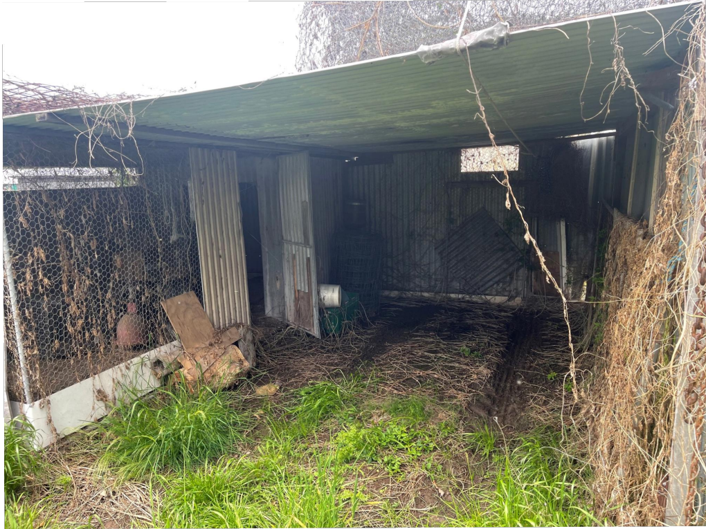
Photo 7: View of the old chicken shed in the centre of the Site. Taken on 7/10/2022.
