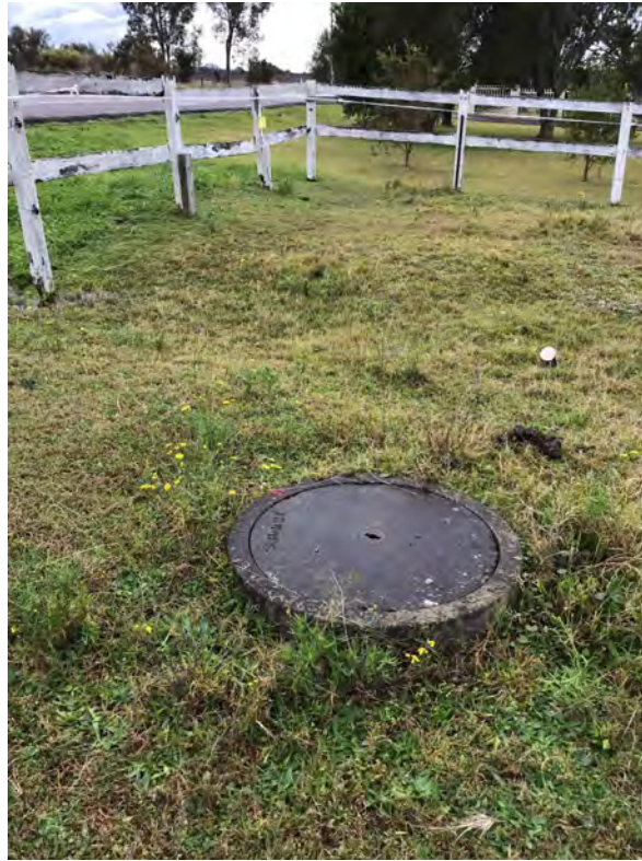
Photo 1: View of Sewer manhole in the northern portion of the Site (facing north)
